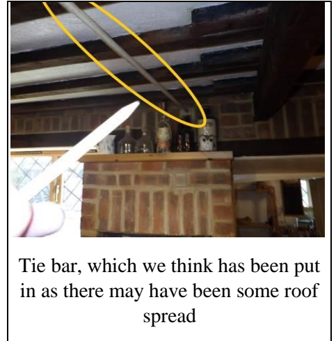
Opening up of wall, which we think will be affecting the roof
