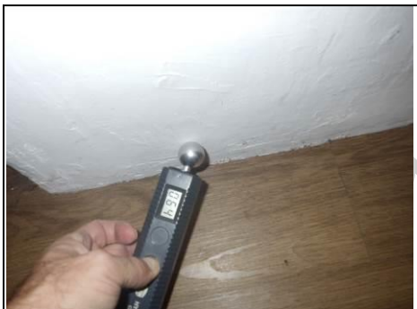
High damp reading in hallway
