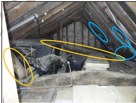
Damp to timbers and extra supports added
