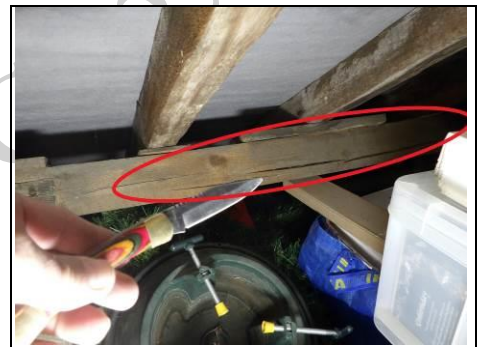
Split in purlin
