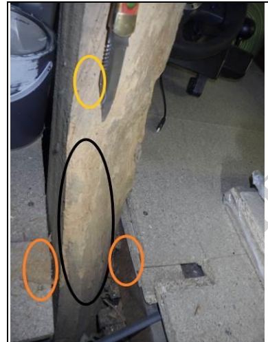
More signs of wood destroying insects
