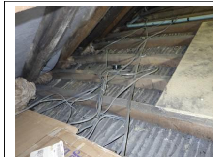
Oldish wiring and Bakelite fitting in kitchen/utility roof
