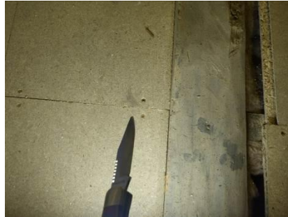
Signs of wood destroying insects to timbers. Our view was very limited due to the screwed down floorboards
