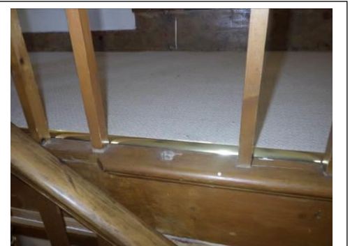
Missing newel posts to stairs
