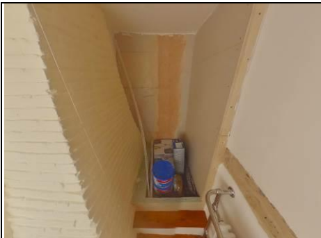
Unfinished shower in first floor en-suite shower room
