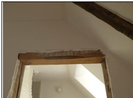
'Lintel' that is not actually a lintel over the en-suite shower room door
