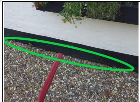
Moss growing to base of wall due to dampness
