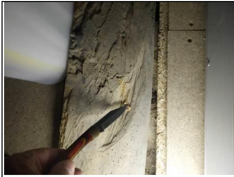
Frass from wood destroying creatures
