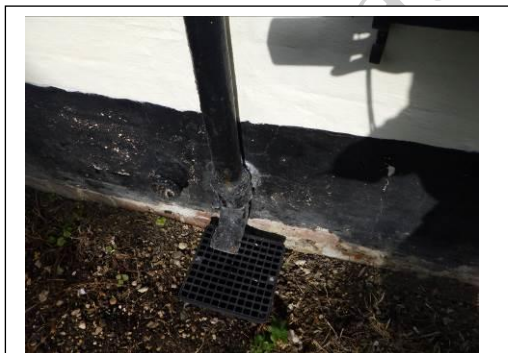
Downpipe discharging quite high, close to property
