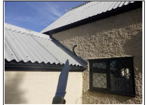
Other side of tie bar
