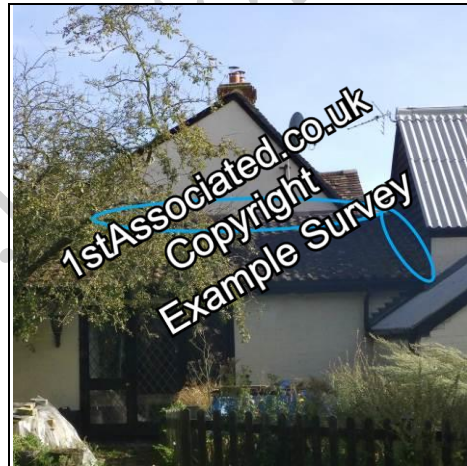
Tile on edge flashing to right side roof
