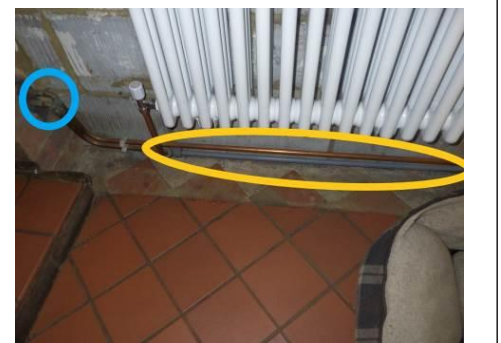
Mixture of copper and plastic pipework to radiator and possible leak
