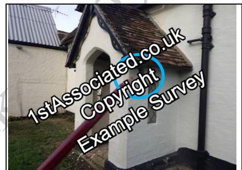
Downpipe on rear porch cut short
