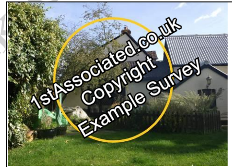
Old photo of what used to be the right gable, which has now been built in front of
