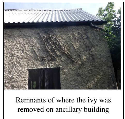
Google photo – ivy removed
