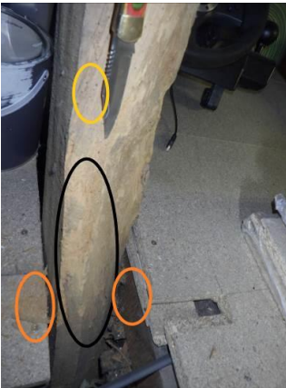
Signs of damage from wood destroying insects in main roof
