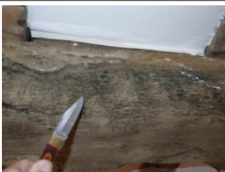
Signs of historic damage (as is often the case) in lounge from wood boring insects
