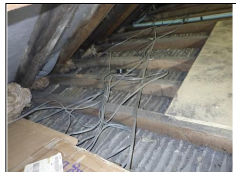
Old electrics in main roof including Bakelite
