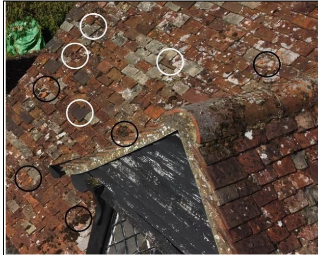
Slipped, displaced, broken and spalling tiles
