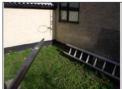
Crack where kitchen building meets pantry/store
