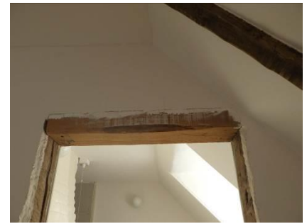
The lintel that is not a lintel over shower room door
