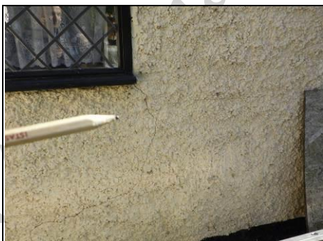
Crack to rough cast cement render on kitchen wall
