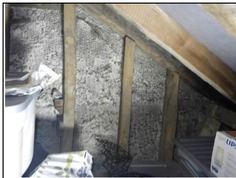
Chicken wire and cement to right side – generally post war to about 1970s
