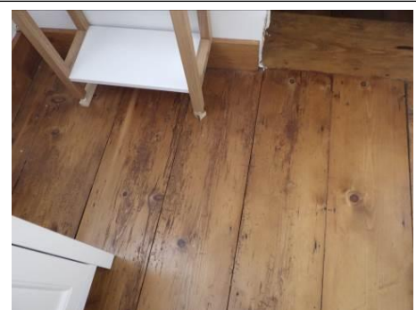
Signs of historic wood destroying insects to floor in lounge
