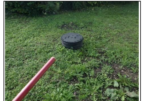
Manhole sticking up is a trip hazard
