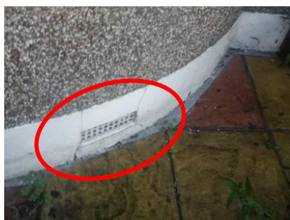
Cracking around air vent to front bay
