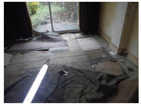
Dampness and deflection in through lounge to rear
