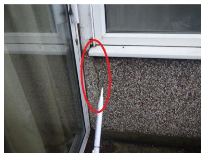
Cracking around rear right lobby
