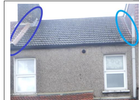
Roof to rear where there have been new tiles on left side (blue) and dampness getting in to rear right (purple) (all directions given as you face the property from the front)
