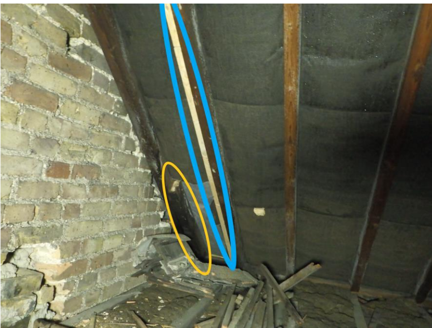
Felt and newish batten (blue), with replacement common rafter foot (yellow)
