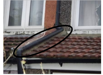
Cement around rear right bedroom
