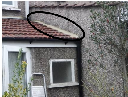
Cement flashing to rear left
