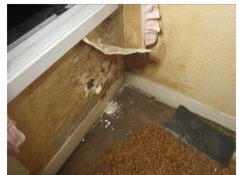
Dampness coming in around rear right bedroom window
