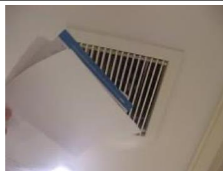
Testing the extract fan which in this case had poor extraction
