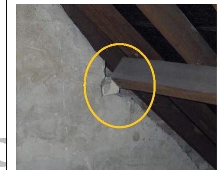
Purlin needs to be monitored
