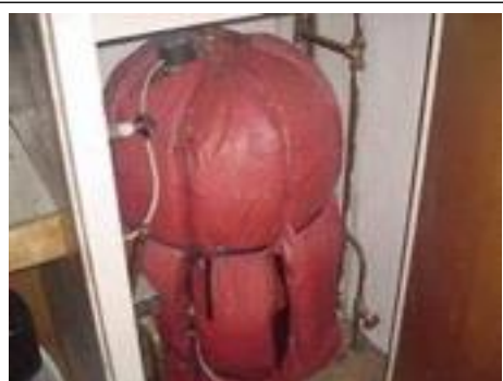
Older style cylinder with loose insulation jacket
