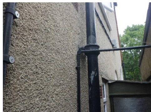
Cast iron soil and vent pipe to left
