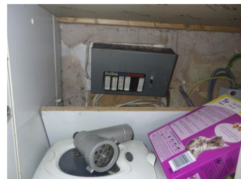
Old fuse board in kitchen cupboard
