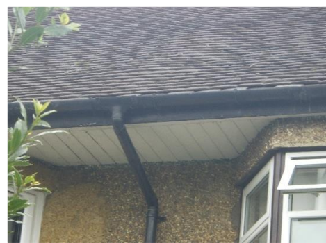
Rear tiles deteriorating
