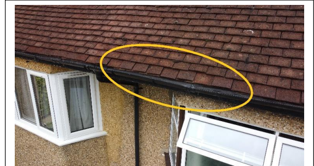
Loose tiles to rear right ~ Aerial View ~
