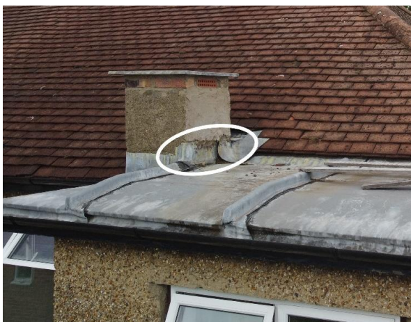
Poor rendering to rear chimney and flashing coming away ~ Aerial View ~
