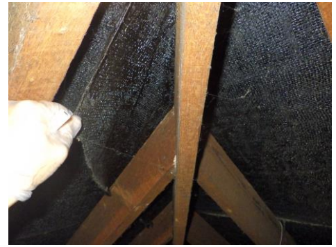
This photo shows the common rafters (the ones that form the pitch of the roof) and area between is the protective underlayer.
