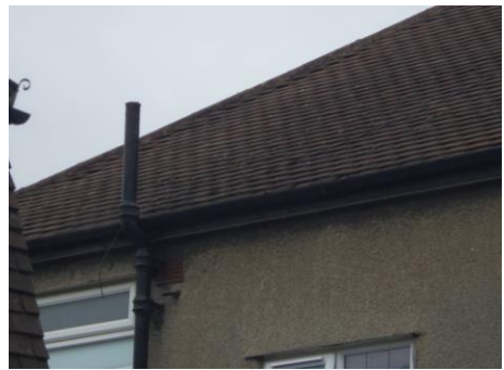
Soil and vent pipe
