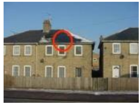
Inappropriate double glazed windows change the look of the property Red circle is insulated roof indicated as snow is not visible
