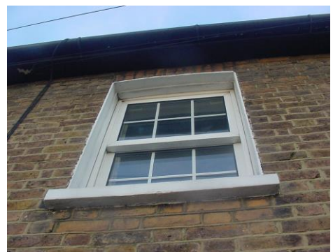
Sliding sash windows can swell in the winter months
