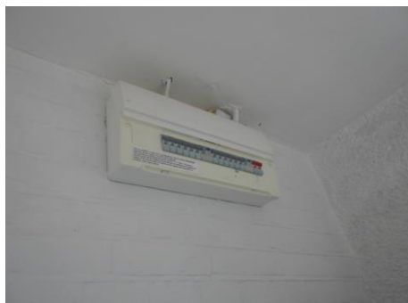
Fuse board in entrance hall
