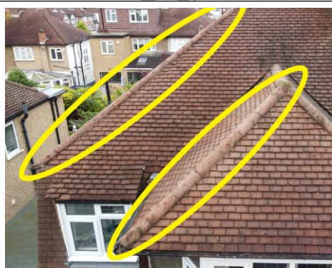
Hairline cracking to the hip of the roof
