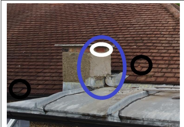
Rear roof Black – sample of slipped or damaged tiles Chimney poor rendering and airbrick ~ Aerial View ~
