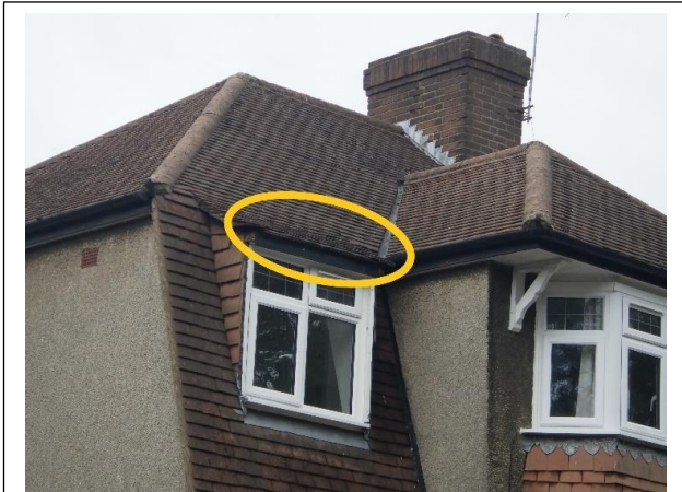
Front tile problems ~ Aerial View ~
