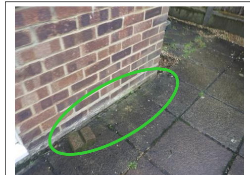
Mould around the base of the single storey extension to rear
