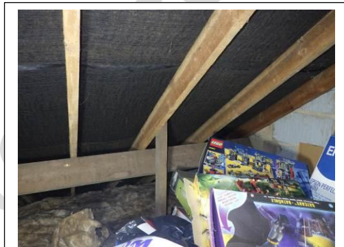
This photo shows the common rafters (the ones that form the pitch of the roof) and area between is the protective underlayer.
