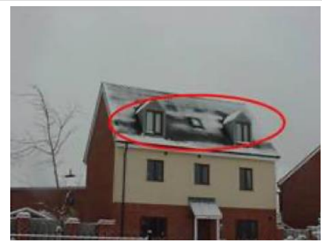
Heat loss via poorly insulated roof
