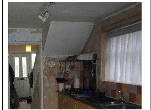
Air filter over cooker but no extraction in kitchen noted
