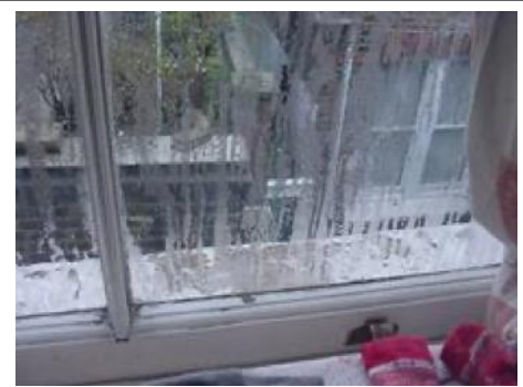
Condensation on window
