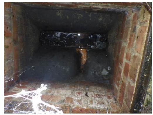
Front manhole blocked
