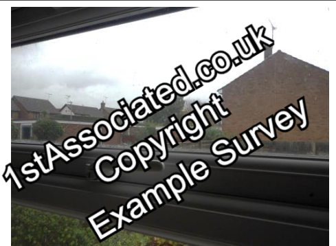
Condensation occurring to end window in kitchen
