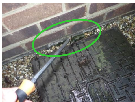
Mould next to building on rear left side
