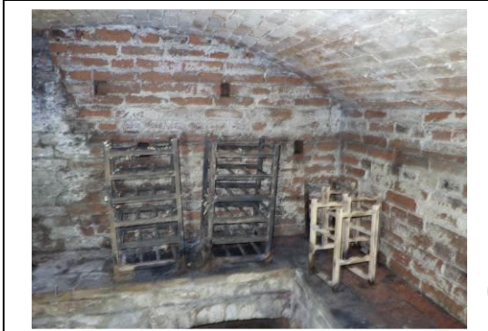
Off ground storage, indicating cellar possibly gets damp
