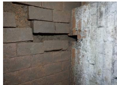
Openings in brickwork which may have been some kind of timber frame (conjecture)
