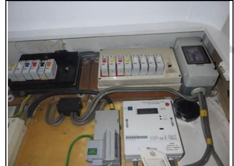
Dated fuse board
