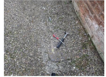
Unable to lift Manhole Three
