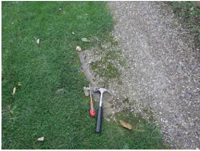
Manhole one to front of right side drive, with bent cover
