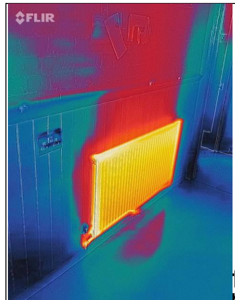
Red shows heat from single panel radiator (Not your property)
