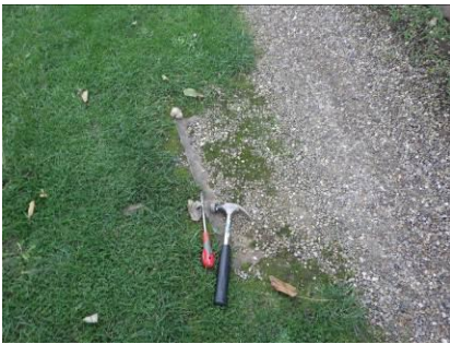
Manhole One to front of driveway has been bent so we were unable to open
