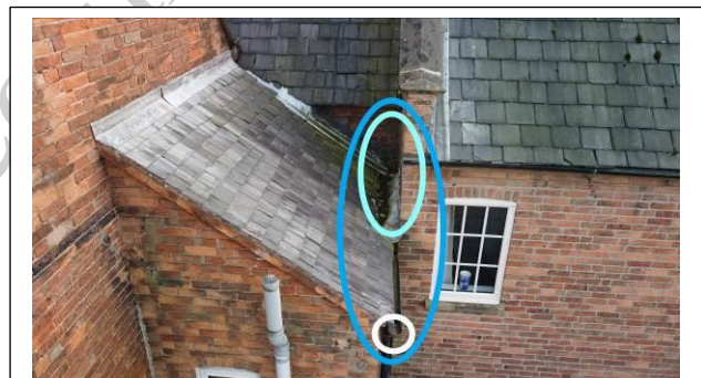
High level rear awkward valley gutter against wall, which looks to be affecting the next door neighbour
