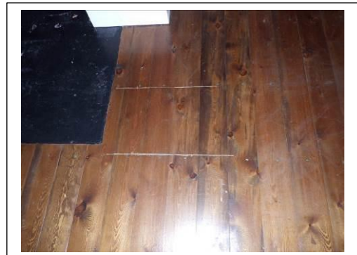
Area of floor in dining room which looks as though it has been opened up before
