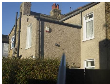
Crack to rear render
