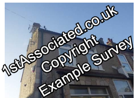
Render and stonework could be hiding cracking
