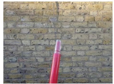
Crack to gable end
