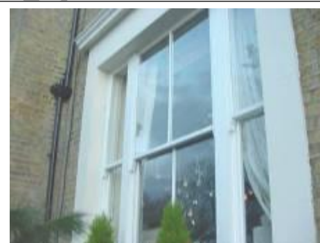
Sliding sash windows can swell in the winter months
