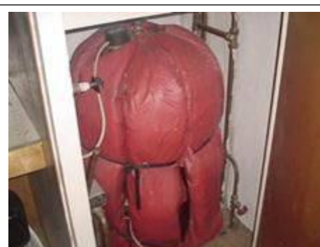
Older style cylinder with loose insulation jacket
