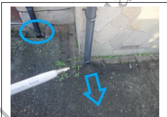
Gutter discharging directly onto the ground and also into a gully
