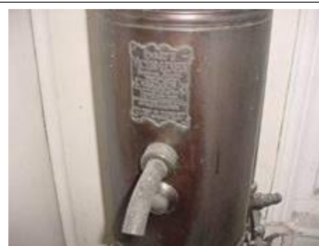
Very old Victorian water heater
