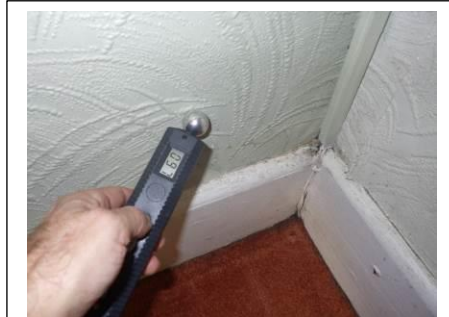
High damp meter reading of 97
