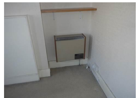
Dated fuse board under stairs
