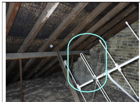
Dampness to front chimney
