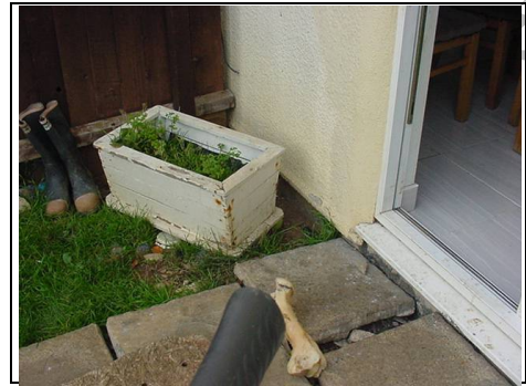
Uneven paving slabs
