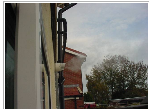
Steam from boiler
