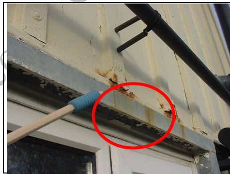
Close up of detail where profile metal sheet meets the lower part of the building
