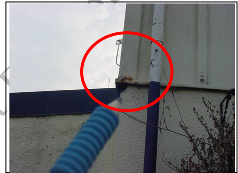
Rust on sill between profile metal sheet and render
