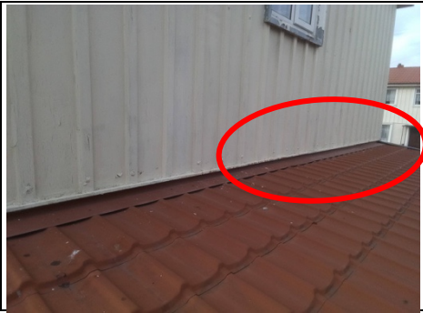
Rusting to rear left
