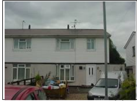
BISF house with a profile metal roof, (again has asbestos roof been removed?), plastic cladding at first floor level (is there insulation between the profile metal sheets and the plastic cladding that is causing condensation) with pebbledash render at ground floor level and modern double glazed windows
