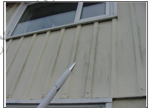
Blackening within panels
