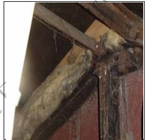
Steel frame visible on a close inspection to the property which is why this is a BISF or non-traditional property
