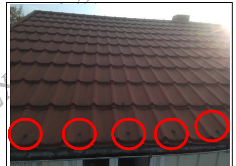
Rusting of anchor bolts
