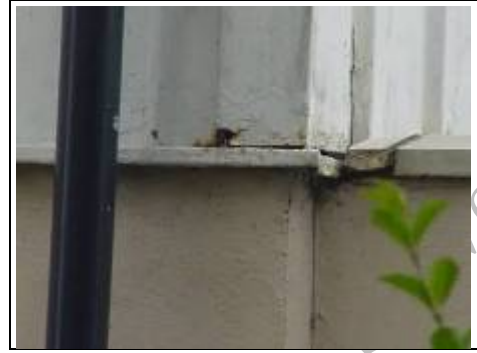
Rusting to profile metal cladding
