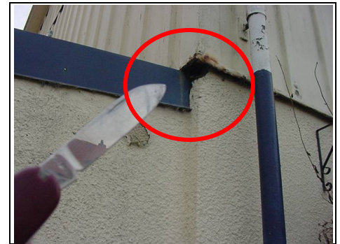
Rusting to sill detail to front left
