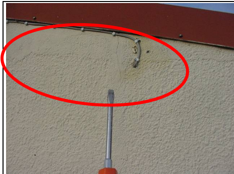
Signs of cracking covered up to rear left
