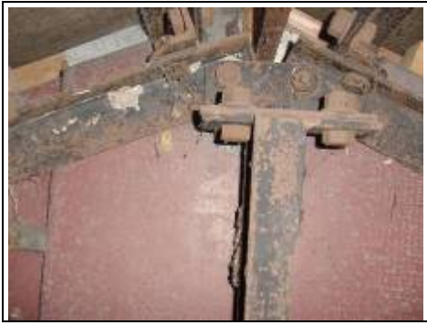
Rusting to a lightweight metal frame or damage or deterioration to the metal frame of a non-traditional house
