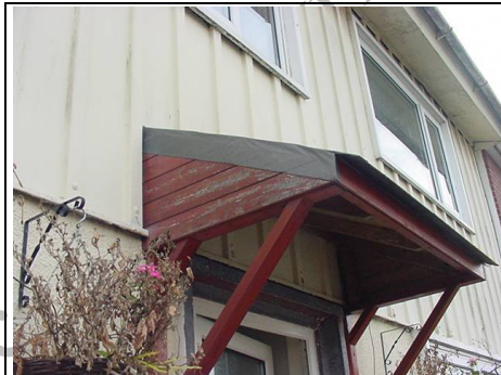
Canopy gallow brackets with flashband on side and timber needs redecoration
