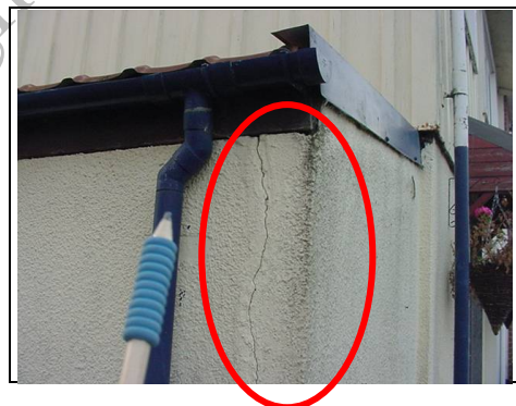
Vertical crack to single storey lean-to
