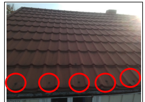
Rusting of anchor bolts
