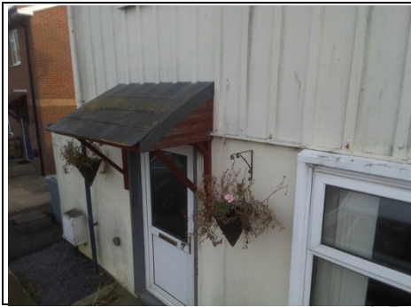
Entrance canopy felt covered
