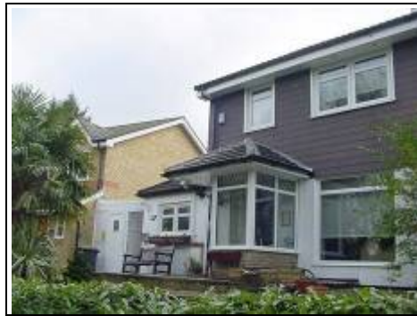
Metal frame house with profile metal sheeting at top and render at bottom. Roof has been changed.
