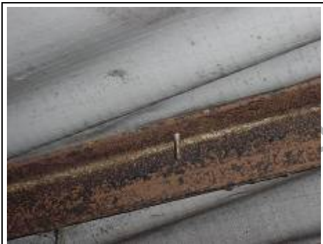
Example of rusting that we have seen in the roof of a metal framed building
