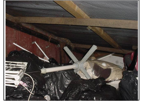
View of roof restricted by stored items
