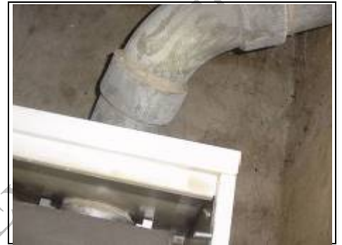
Example of Asbestos flue on similar metal frame non traditional property (Not your property)
