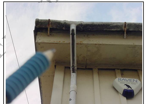
Rusting at high level to fascias
