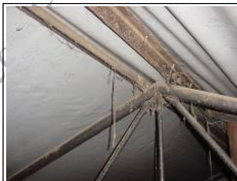
Example of tubular metal frame within the roof of a metal framed property
