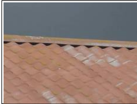
Weathering effect to roof
