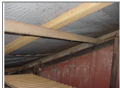
Rust to metal frame
