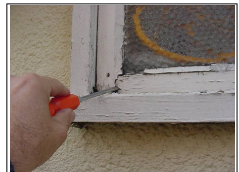
Timber window in need of work
