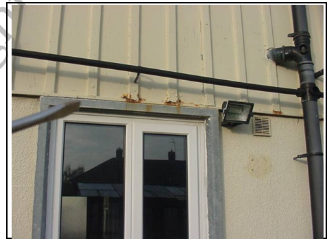
More support required to pipework
