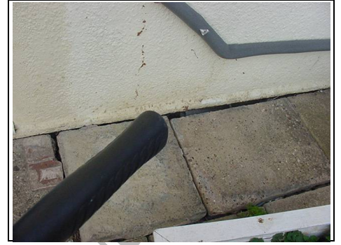
Rear paving slabs uneven
