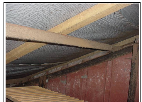
Rust to metal frame
