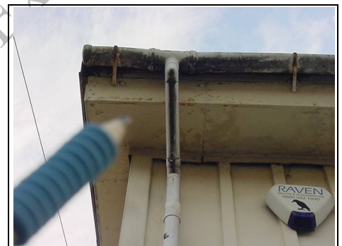
Fascias and soffits possibly asbestos
