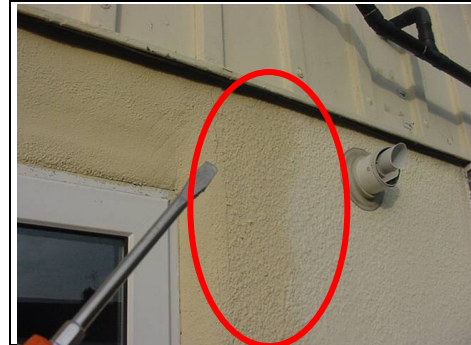
Vertical crack to rear
