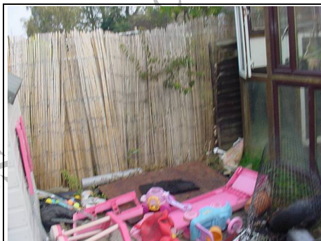
Left fence in need of repair
