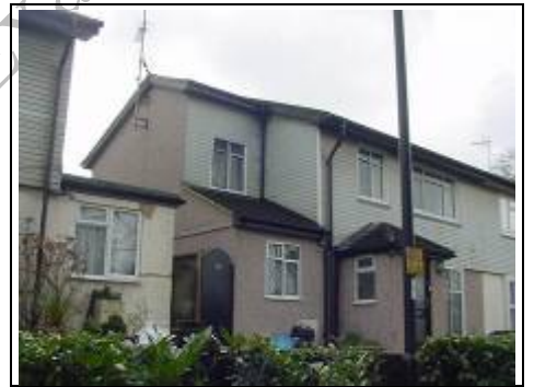
Pebbledash render in parts as well as plastic cladding and extensions but again the main part of the building is still a metal frame
