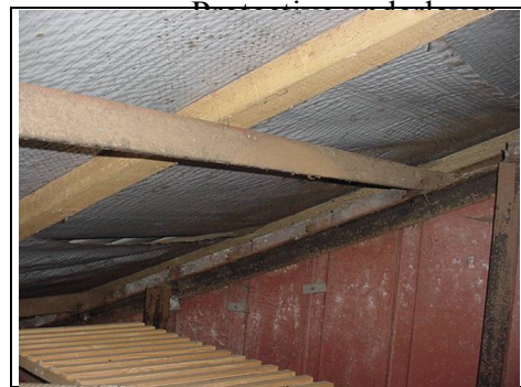
Rust to metal frame
