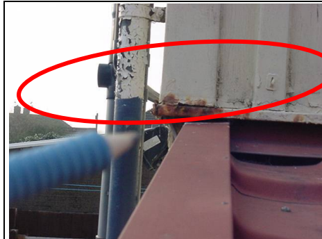
Rust to rear left corner
