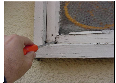
Timber window in need of work
