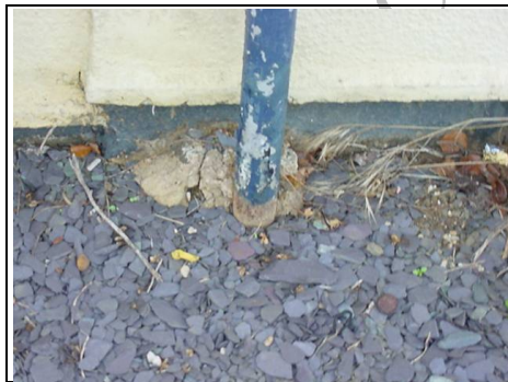
Downpipes feed directly into ground
