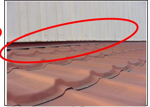
Rust to sill detail of single storey extension
