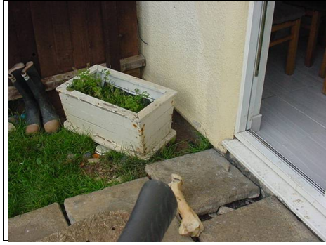
Uneven paving slabs
