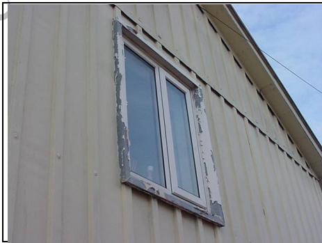
Deterioration to left window
