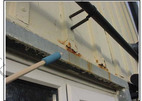
Rust where profile metal sheet meets the lower part of the building
