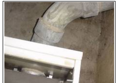
Example of Asbestos flue on similar metal frame non traditional property (Not your property)
