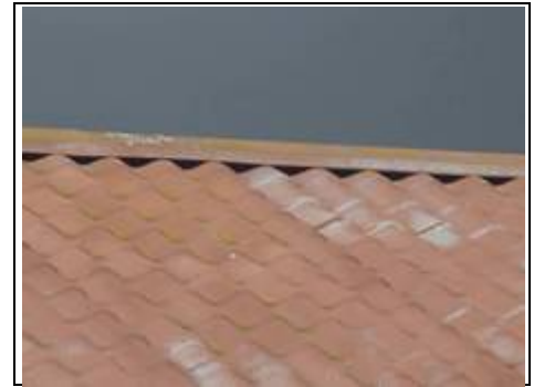
Example of weathering to profile metal roof (Not this property)
