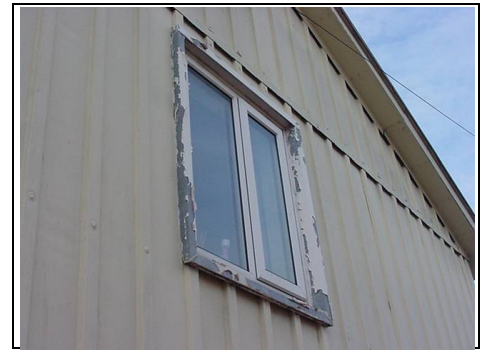
Deterioration to left window surrounding metal frame
