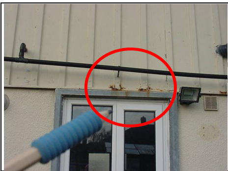
Rusting to drip detail where profile metal sheet meets render and window surround
