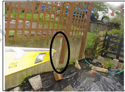
Crack in front left side retaining wall
