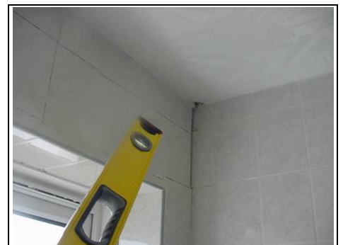
Black mould in bathroom
