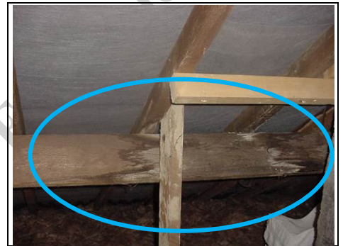
Dampness to timbers
