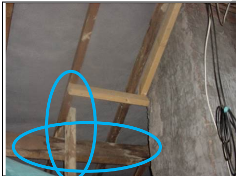
New timber visible and dampness to timbers around chimney
