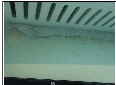
Close up of damage to render (client's photo)
