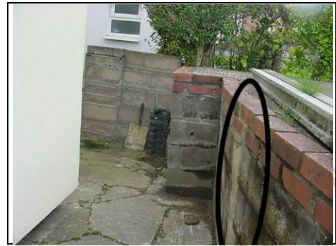
Crack to right side retaining wall around drop from front driveway it
