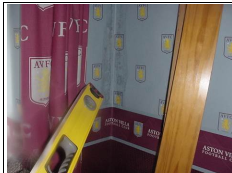
Black mould to corner of rear right bedroom
