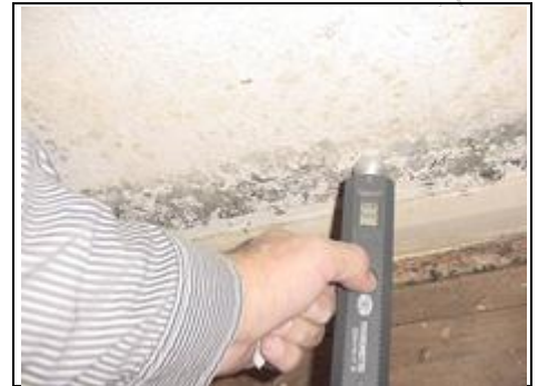
Black mould and high damp meter readings
