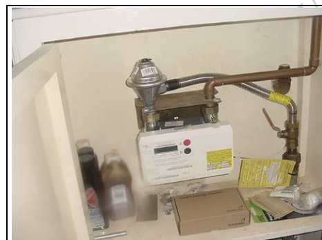
Gas meter in kitchen
