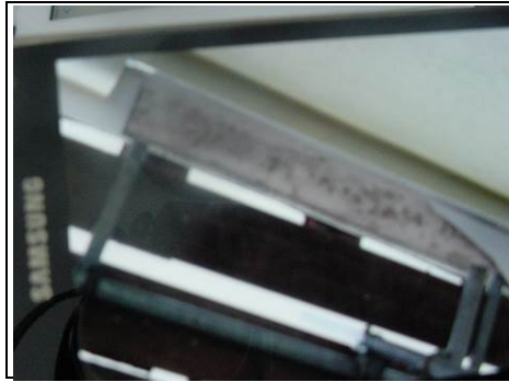
Deteriorating timber fascias board
