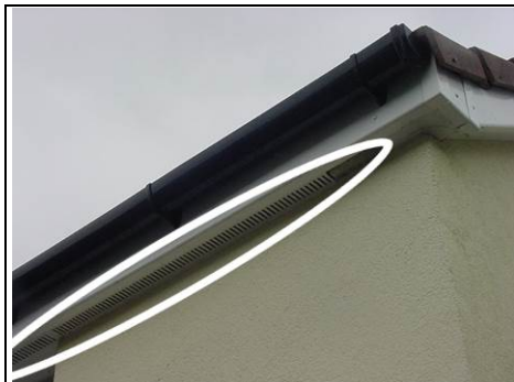
Plastic soffits with vents fitted in many short sections
