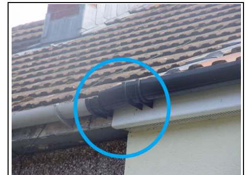
Awkward detail to front where the guttering meets next door's gutter
