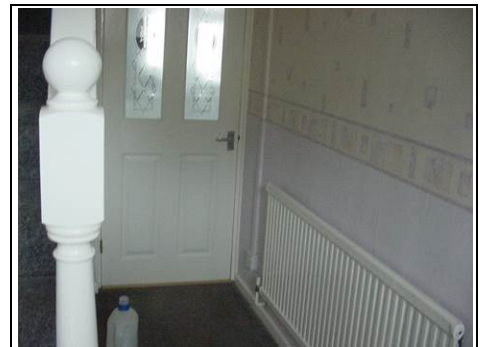
Single panel radiator in hallway
