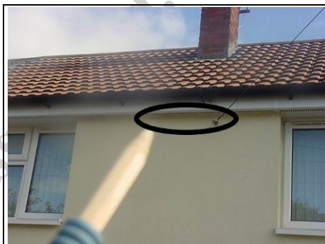
Damage to external wall
