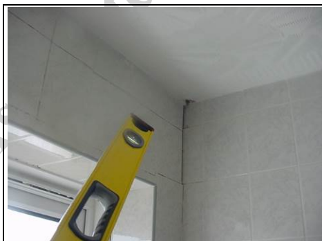
Black mould to corner of wall
