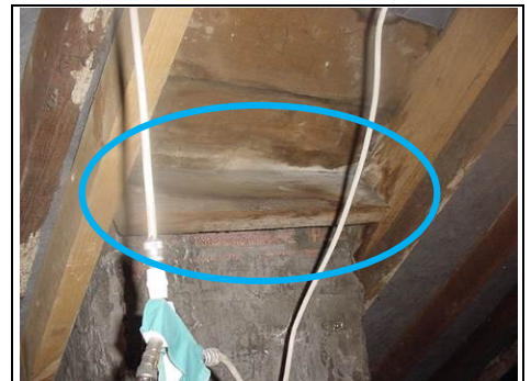
Dampness on timbers around chimney
