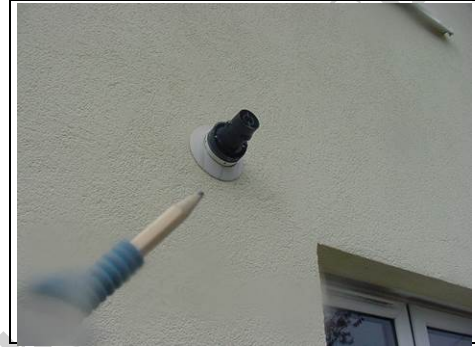
Flue for boiler
