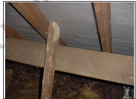
This photo shows the common rafters (the ones that form the pitch of the roof) and the light area between is the underlayer.
