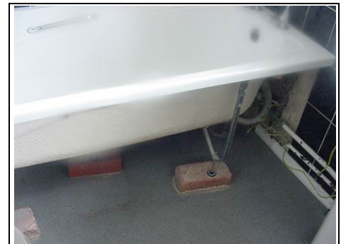
Bath panel missing
