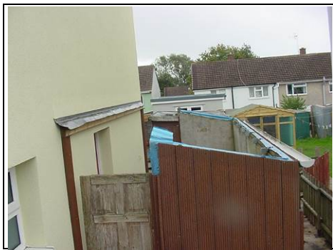
Half-built lean-to to right side of property
