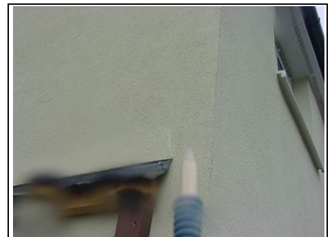
Slight hairline crack just above the flashing
