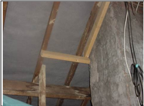
Water damage around chimney
