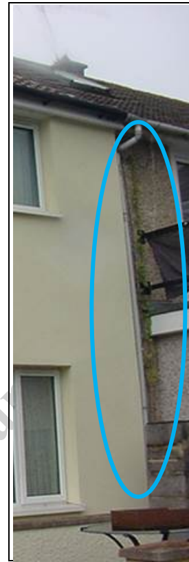
Rear downpipe on next door's property with long run of gutter
