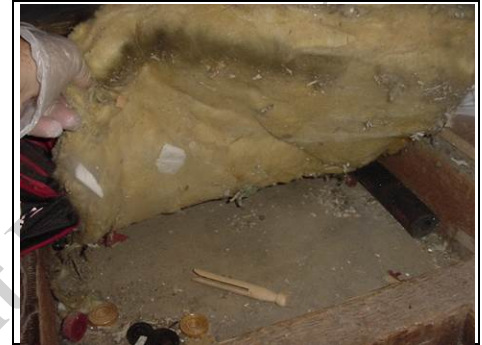
Plasterboard or proprietary boarding noted in roof space
