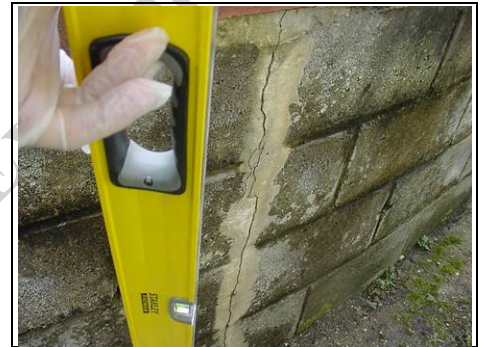
Close up of crack
