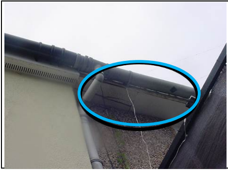
Rear downpipe on next door's property with long run of gutter
