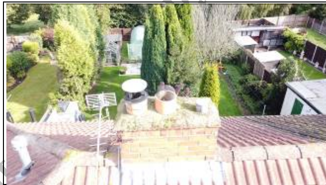
Chimney and flue
