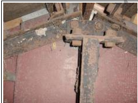
Rusting to a lightweight metal frame or damage or deterioration to the metal frame of a non-traditional house
