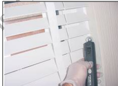
Damp test to reveal of window
