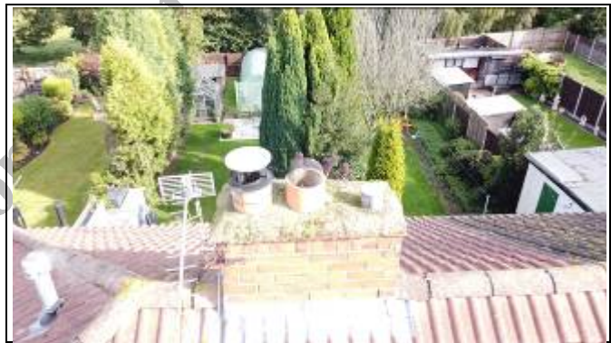
Chimney and flue ~ Aerial View - 360 Photo ~
