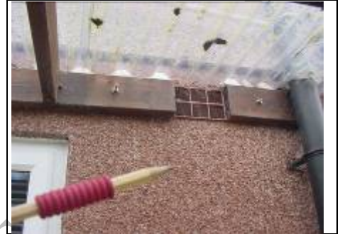
High level air vent
