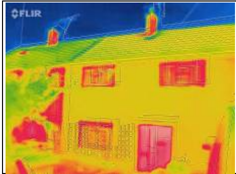
Front of property showing heat coming through windows and door (Not your property)
