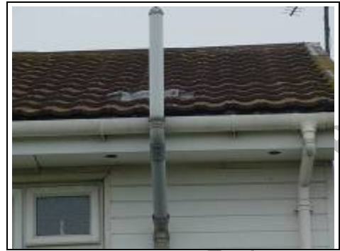
New plastic soil and vent pipe on a non-traditional house
