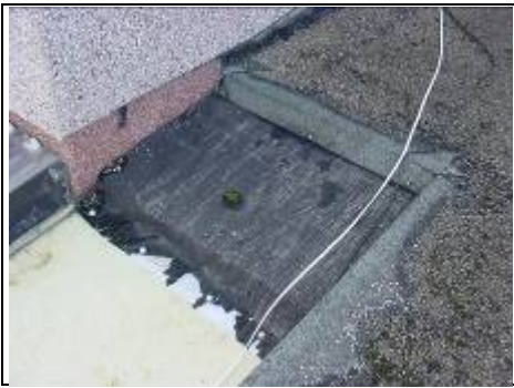
Link corridor roof needs replacing
