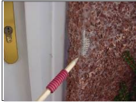
Render starting to deteriorate and reinforcement layer coming through
