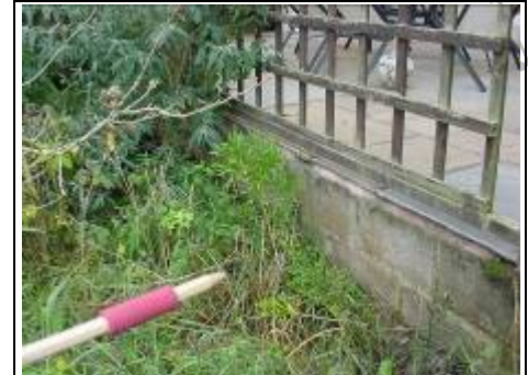
Small retaining wall needs weep holes
