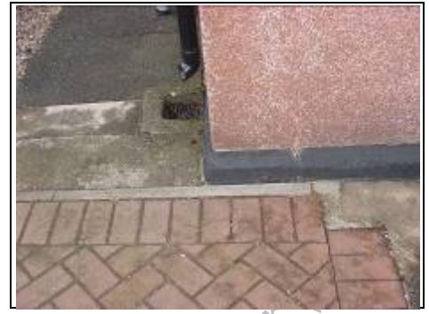
Downpipe and no wall around gully
