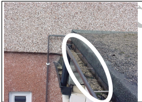
Debris to gutter on outbuilding roof
