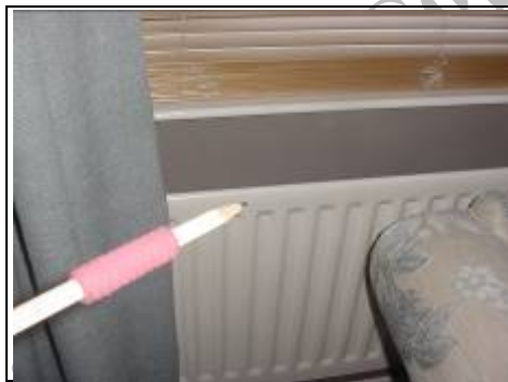
Single panel radiator
