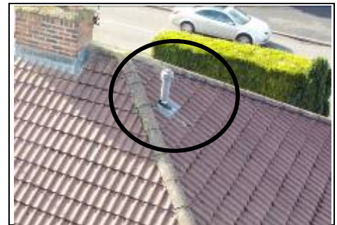
Flue to left
