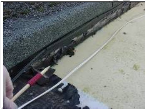
Side detailing where we assume water getting through
