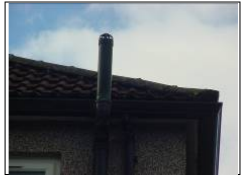
Plastic soil and vent pipe to rear
