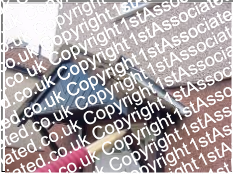
No gutter to front entrance
