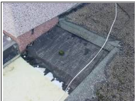
Roof needs replacing
