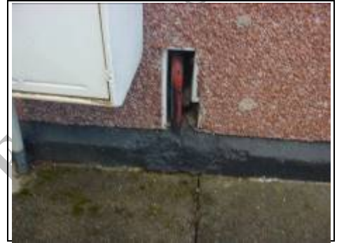
Insulation cut a pipe
