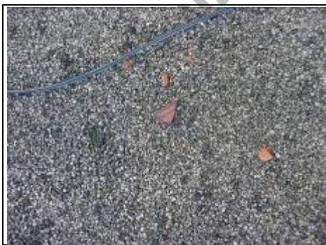
Broken roof tile on flat roof
