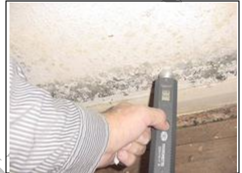
Black mould and high damp meter readings
