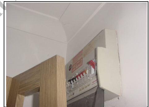
Fuse Board in hallway
