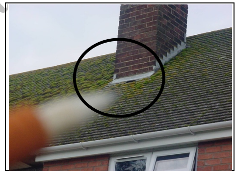
Tile missing at base of chimney
