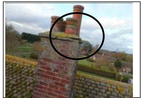
Chimney needs repair
