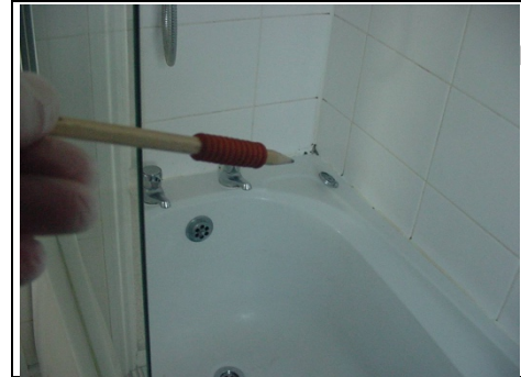
Black mould in bathroom
