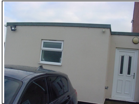
No window drip
