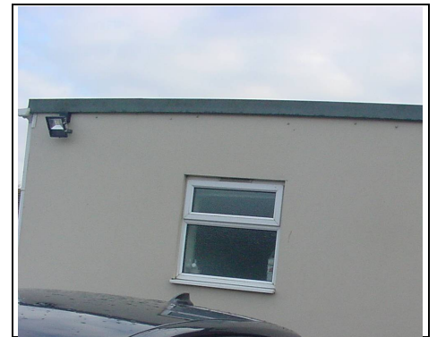
Outbuilding window with no trickle vents
