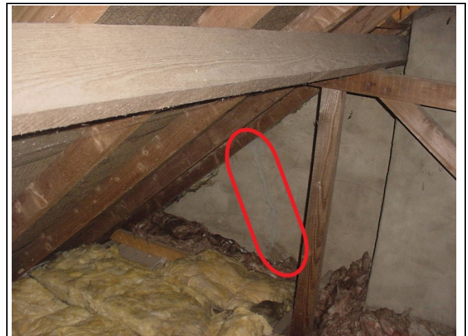
Crack visible in roof space
