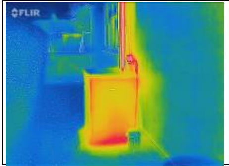
Worcester boiler located externally
