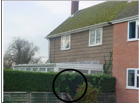
Fence on right side propped up
