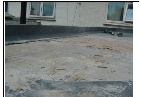
Example of GRP roof with major problems (Not your property)
