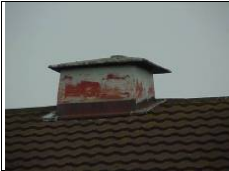
Asbestos original chimney non traditional house
