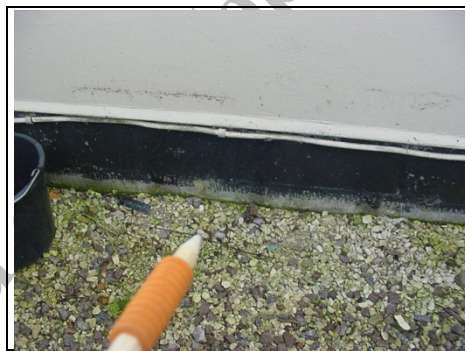
Water sitting to base of outbuilding
