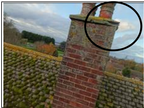
Chimney needs repair
