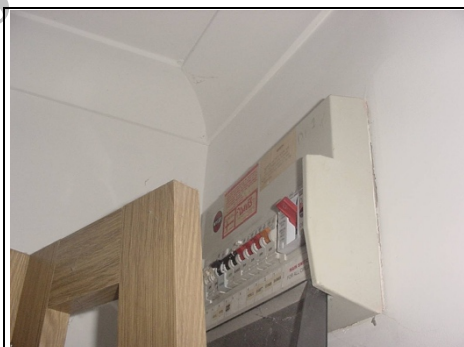
Fuse Board in hallway
