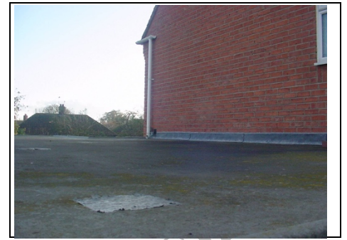
Repair on GRP roof and lead flashing where flat roof meets main building
