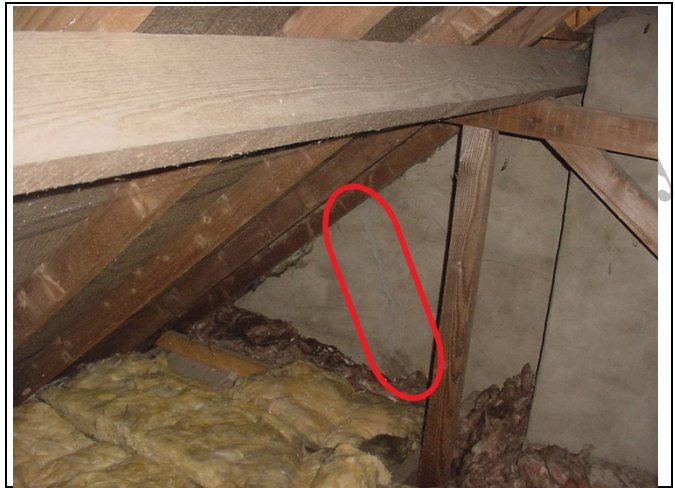
Crack visible in roof space
