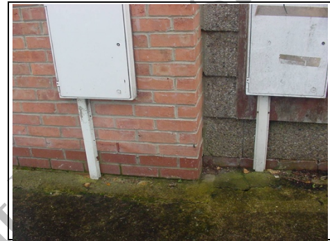
No damp proof course visible
