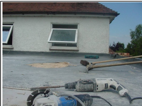
Example of a GRP roof being stripped (Not your property)
