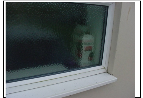
Mould and moss around window
