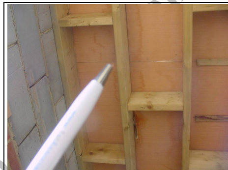
Example of dampness coming through when we stripped back the ceilings (Not your property)
