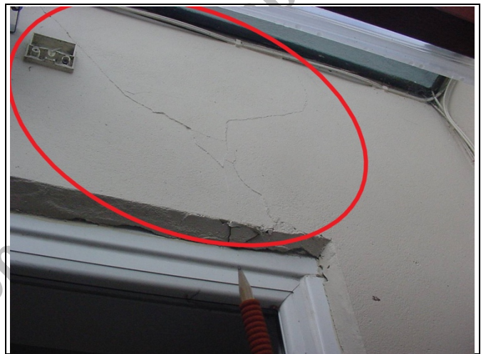
Crack in outbuilding
