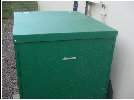
Worcester boiler to side of outbuilding
