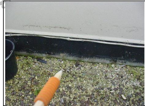
Water sitting to base of outbuilding
