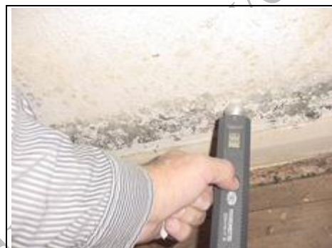
Black mould and high damp meter readings
