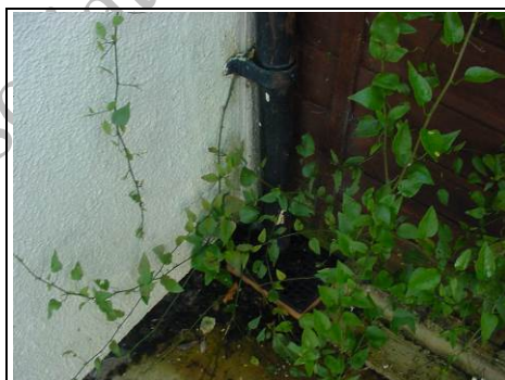
Downpipes feed directly into shallow surface gullies
