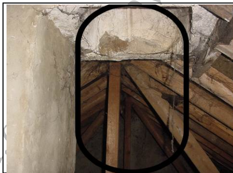
Front of chimney removed in roof space, black oval indicates where that part of the chimney once was
