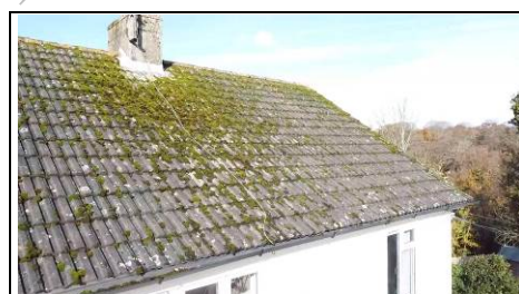
Concrete tiles with moss covering Aerial view – 360 photo
