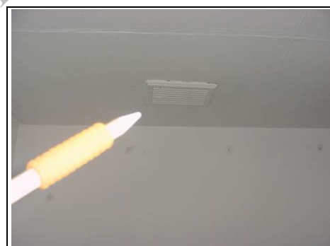
Vent in ceiling
