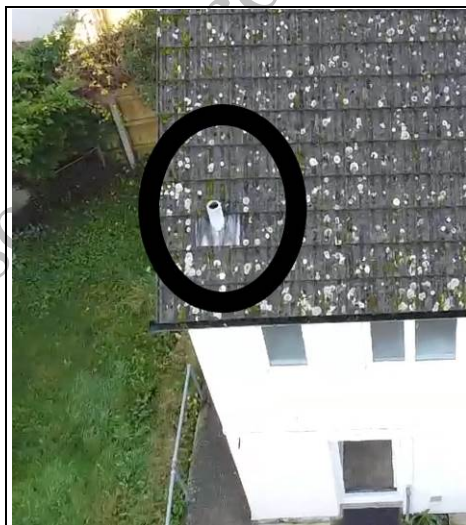
Soil and vent pipe difficult to view but it may be asbestos?
