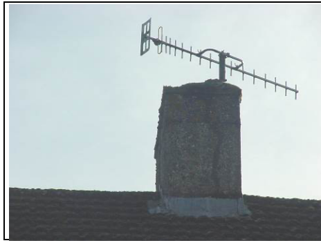
Crack to rear render
