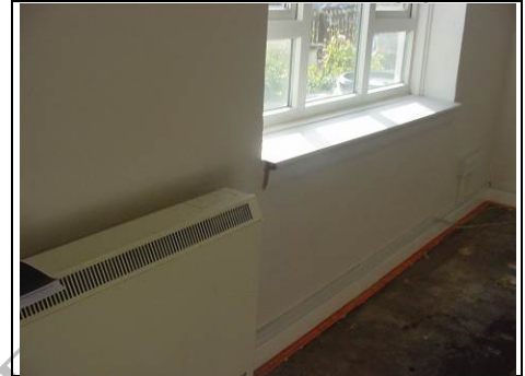
Electric storage heater
