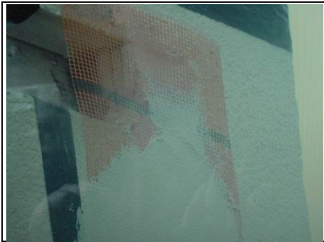
Reinforcement visible (not your property)
