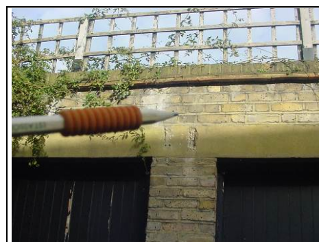
Deterioration to concrete lintel with reinforcement showing through (Not your property)
