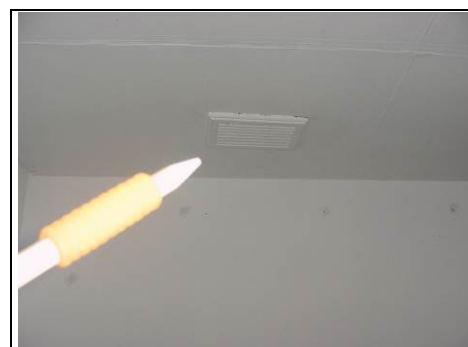
Vent in ceiling
