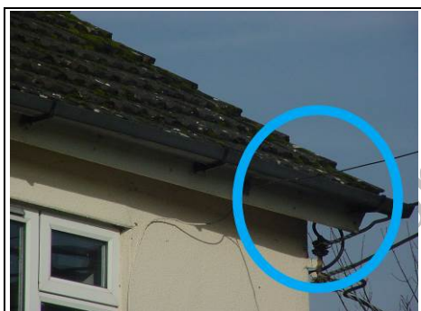
Front right corner, where approximate area of dampness is
