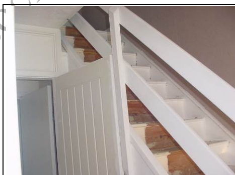
Staircase not up to modern standards
