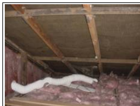
Extract vent to outside often discharges into roof which is essential that they do not in this type of roof
