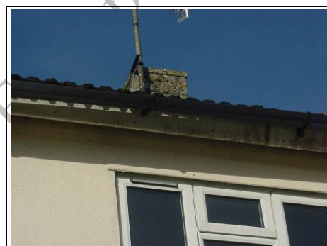
Awkward fascia detail
