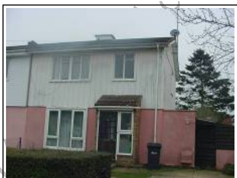
Painted cladding to non-traditional property
