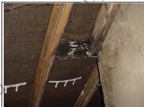
Dampness coming in around chimney
