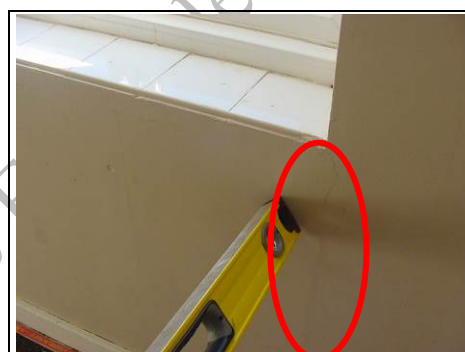
Crack below window
