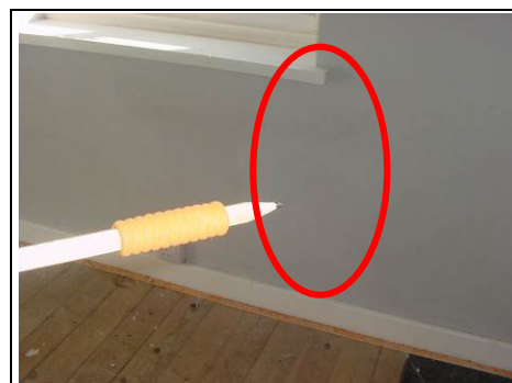
Front right bedroom crack to wall
