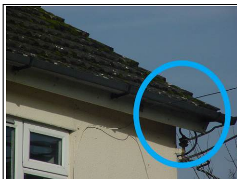
Front right corner, where dampness is
