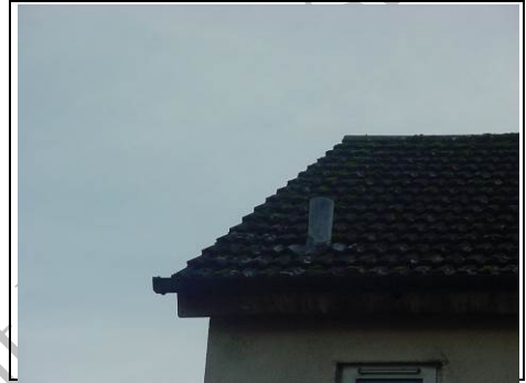
Soil and vent pipe
