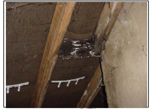
Rot around chimney
