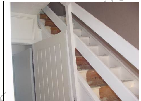
Staircase not up to modern standards
