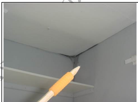
Blackness to corner of front right bedroom, possible condensation, possible roof leak
