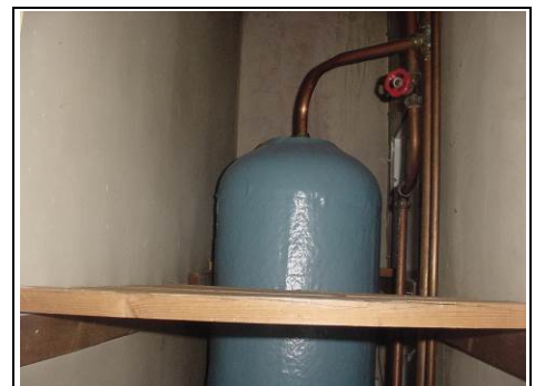
Hot water cylinder
