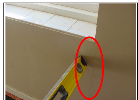
Crack below window
