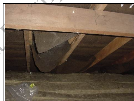
This photo shows deterioration to the underlayer with it hanging it down.
