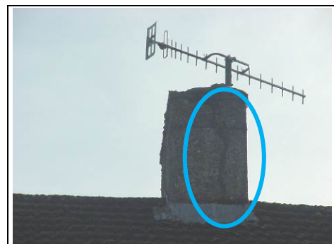
Crack to rear of chimney
