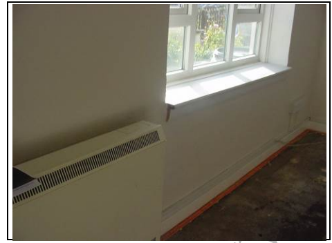
Electric storage heater
