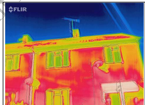
Thermal imaging photo of front of property
