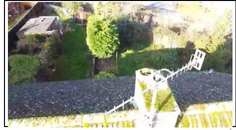
Moss to top of chimney (flaunching) Aerial view – 360 photo flashing
