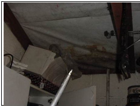
Dampness coming in through garage roof
