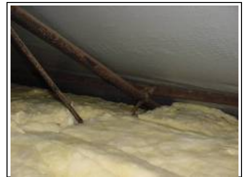
Example of over insulation of a metal framed property which causes condensation
