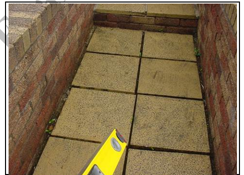
Paving slabs not bedded
