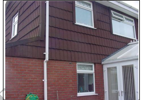
Pressed metal tiles to first floor and brick tiles to ground floor
