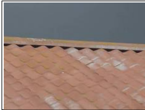
Weathering effect to roof
