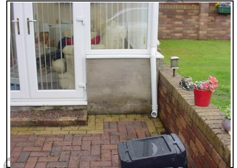
Downpipe by conservatory discharging in wrong area
