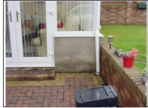
Downpipe by conservatory discharging in wrong area
