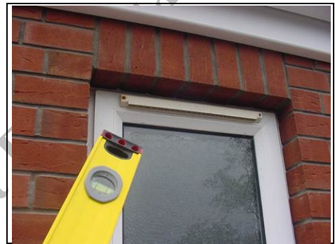
Only trickle vent in the windows is to the ground floor WC
