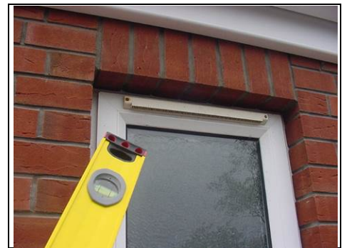
Only trickle vent in the windows is to the ground floor WC
