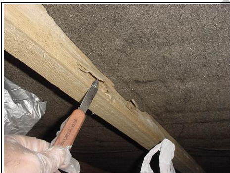
Damaged timber batten in the unlined area of the roof
