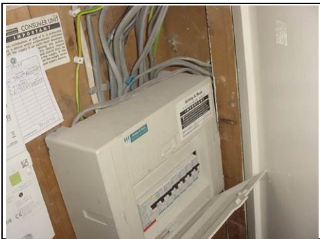
Dated fuse board under the stairs
