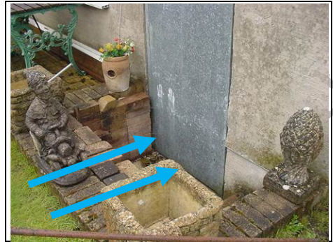
The garage is partially below ground and water will run into this area and then internally
