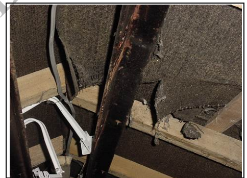
Protective underlayer not bedded particularly well which may have been an area affected by removing the chimney
