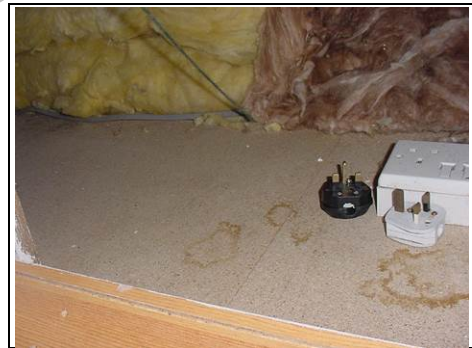
More staining in roof space
