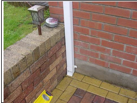
Rear downpipe discharging close to wall
