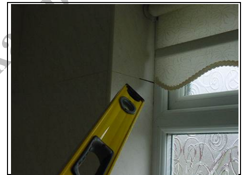
Very slight black mould in bathroom
