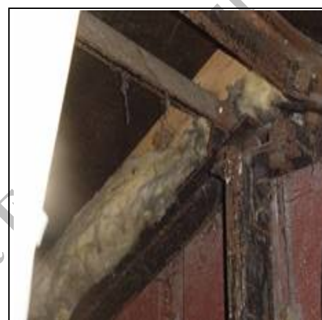
Steel frame visible on a close inspection to the property which is why this is a BISF or non-traditional property
