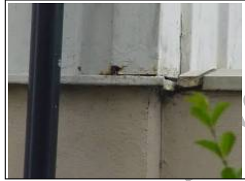
Rusting to profile metal cladding
