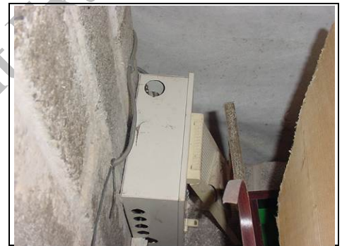
Dated fuse board in garage
