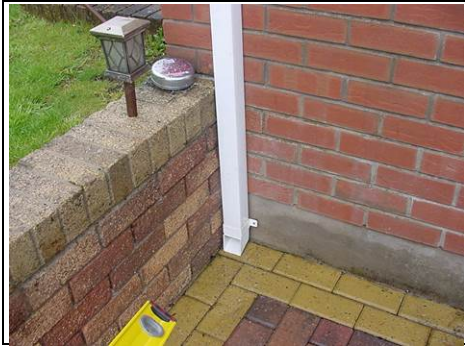
Rear downpipe discharging close to wall
