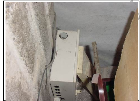
Dated fuse board in garage
