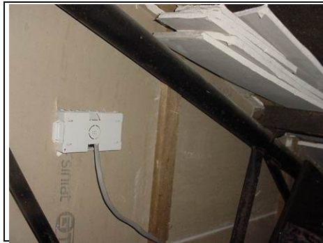
DIY electrics in roof space
