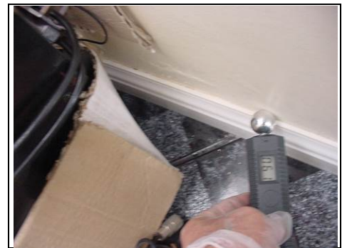
Slightly high damp meter readings in conservatory
