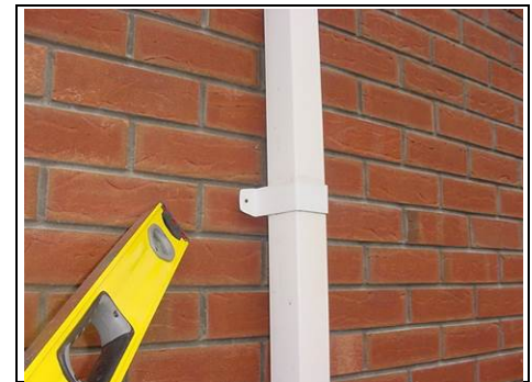
Rear downpipe not fixed
