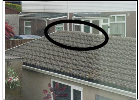
Dip in garage roof to the rear and there may be deterioration in this area
