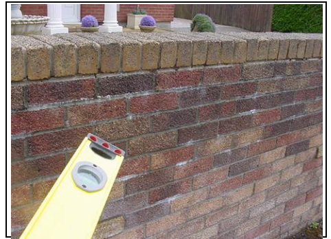
Efflorescence to front brick wall
