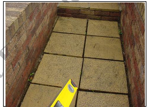
Paving slabs not bedded
