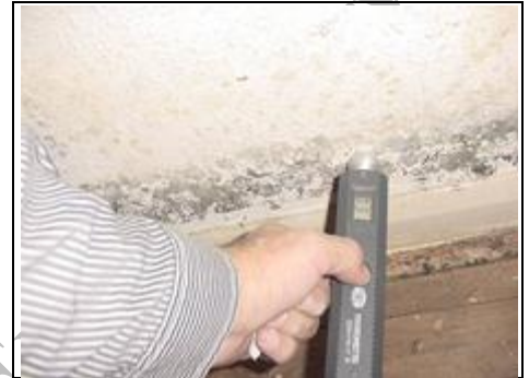
Black mould and high damp meter readings
