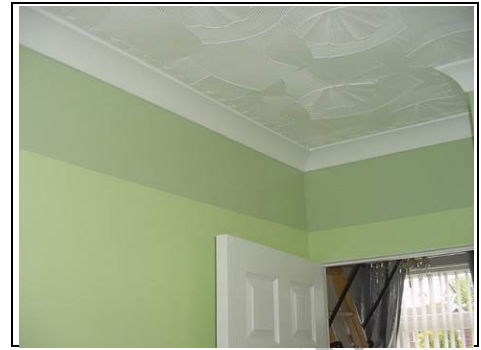
Textured paint in fan pattern
