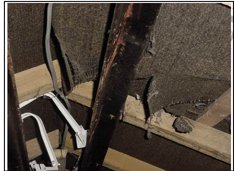
Displacement of protective underlayer
