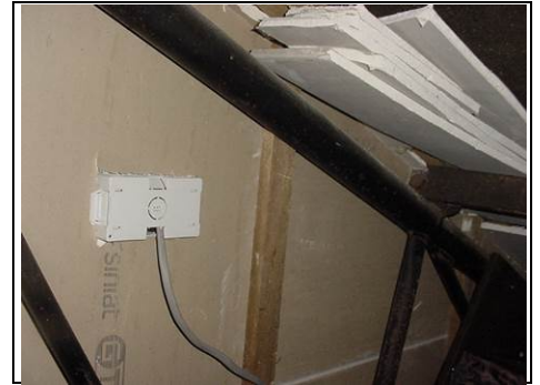
DIY electrics in roof space
