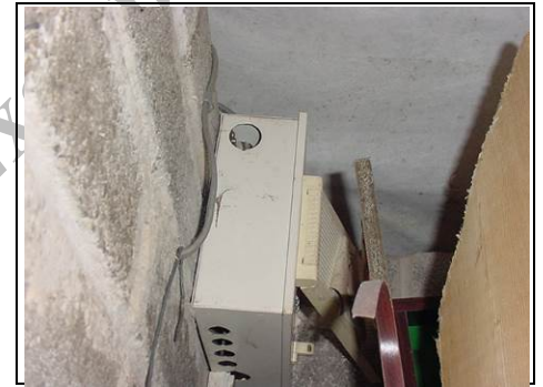
Dated fuse board in garage
