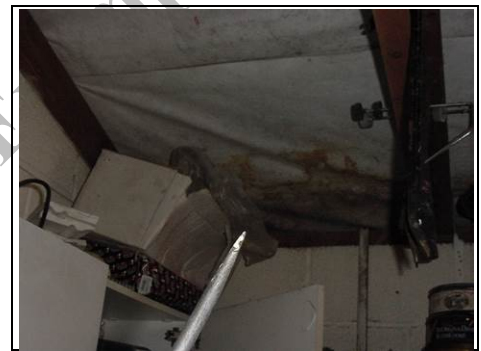
Dampness coming in through garage roof
