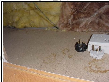
Staining in lined area
