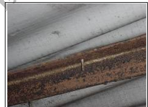
Rusting within the roof between the insulation and plastic protective underlayer
