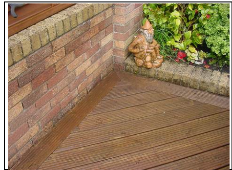
Gaps in decking
