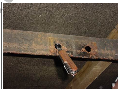
Holes in one of the brackets close to where we believe the chimney used to be
