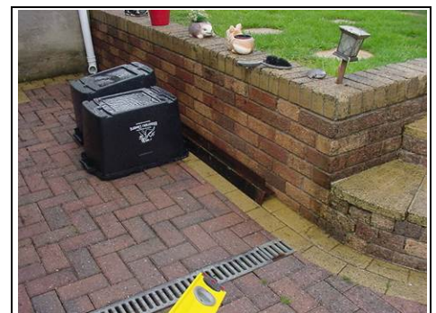
Rear retaining wall needs weep holes adding
