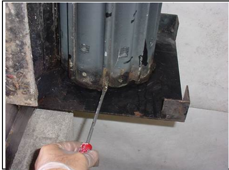
Rusting automatic garage door
