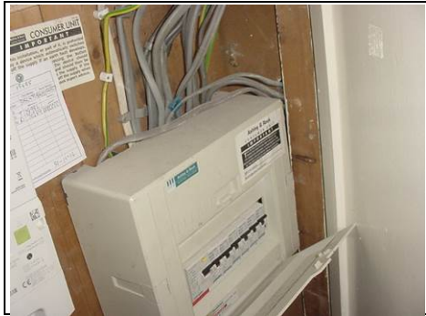
Dated fuse board under the stairs
