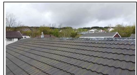
Pressed metal roof, a chimney would have once been present Aerial view – 360 photo
