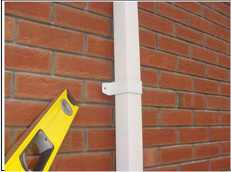
Rear downpipe not fixed properly
