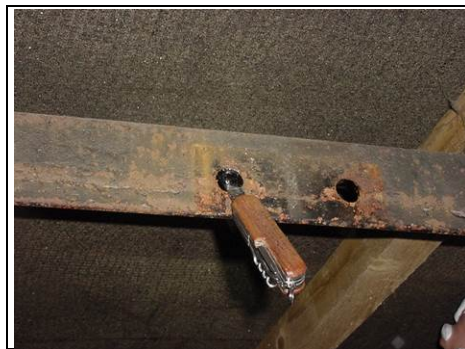
Holes in metal roof purlin which may be where the chimney was once secured
