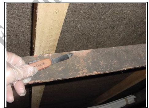
Rust where red oxide is showing through
