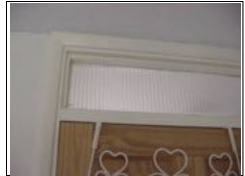
Fluted glass above doors not safety glass
