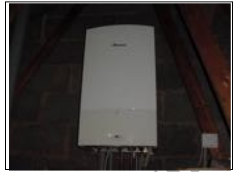
Boiler within roof
