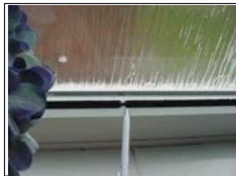
Double glazing rubber seal perished
