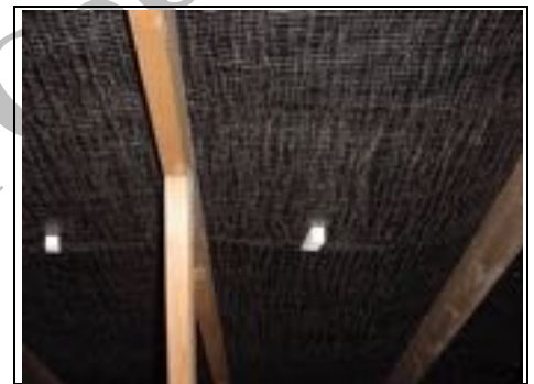
This photo shows the common rafters (the ones that form the pitch of the roof) and the dark area between is the underlayer.
