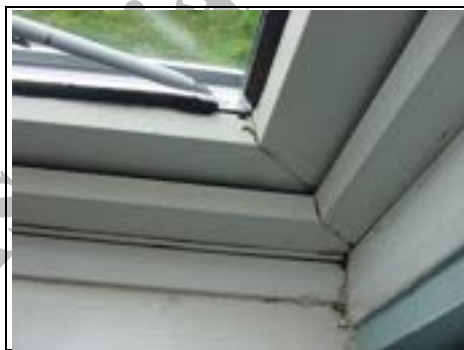
Black mould to windows and rubber seals perishing
