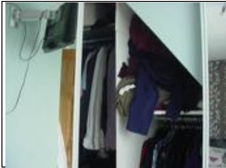
Cupboard underneath the pitch of the roof susceptible to cold bridging
