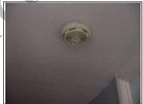
Alarm to be replaced
