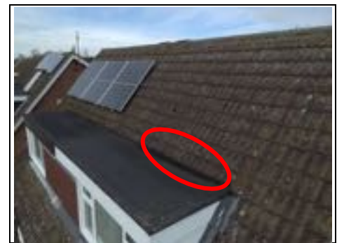
Water tipping/sitting on front flat roof ~ Aerial View - 360 Photo ~
