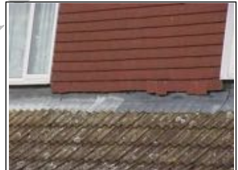
Slipped vertical tiling to dormer
