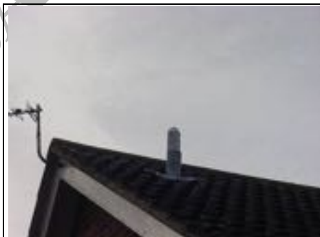
Soil and vent pipe
