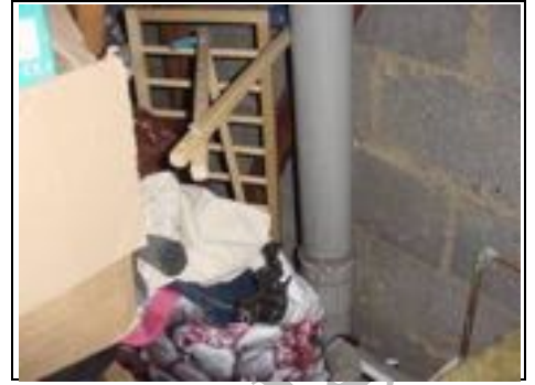
Clothes stored within roof space
