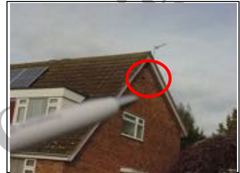
Flue from boiler within roof
