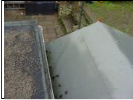
Garage – water discharging on end gutter
