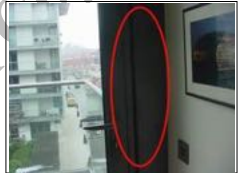
Condensation visible on metal return of window
