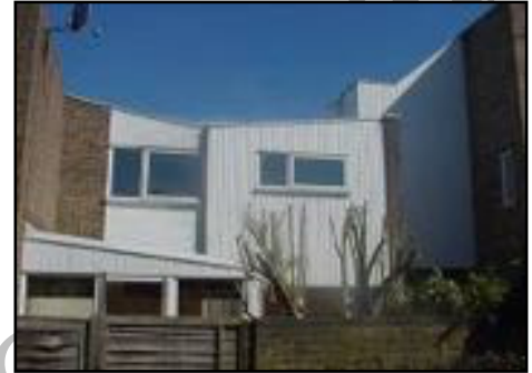
1970's property with cold bridging to the roof beams and the lintels
