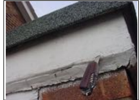
Rot to garage fascia
