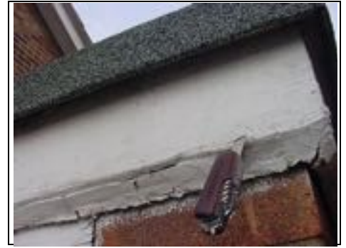
Rot to garage fascia
