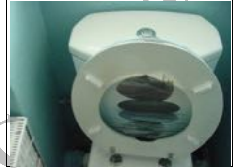
Damaged toilet seat
