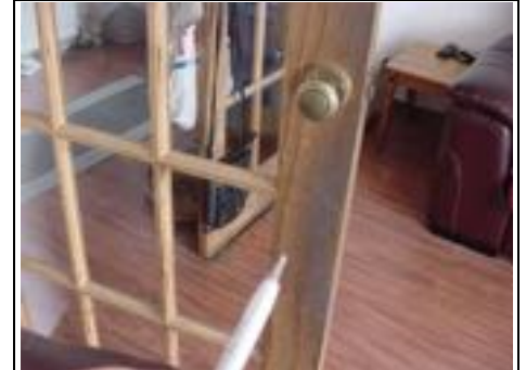
Glazed door worn
