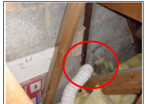
Extract from bathroom discharging into roof
