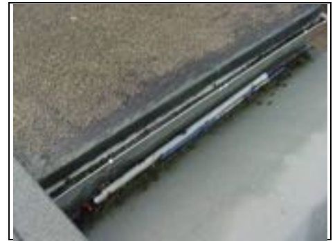
Garage gutter overflowing onto shed
