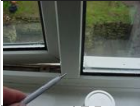
Condensation in rear right bedroom
