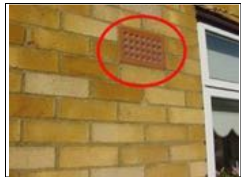
Air brick may not ventilate room enough
