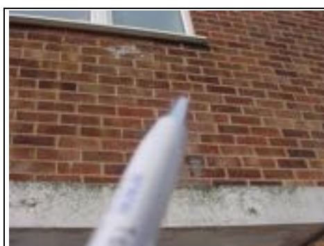
Circular cement fillets where insulation added and/or wall ties
