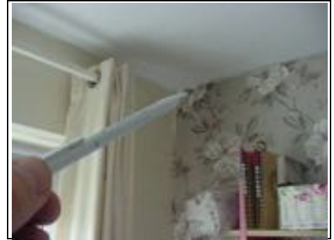
Black mould painted over in rear right bedroom
