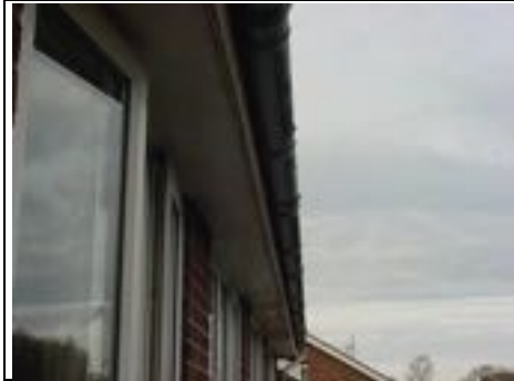
Deterioration to fascias and soffits of the house
