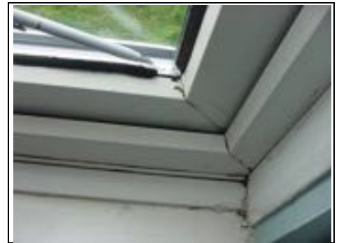
Black mould to windows and rubber seals perishing
