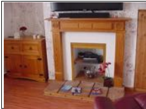
Front fireplace with asbestos flue – do not use unless new chimney installed
