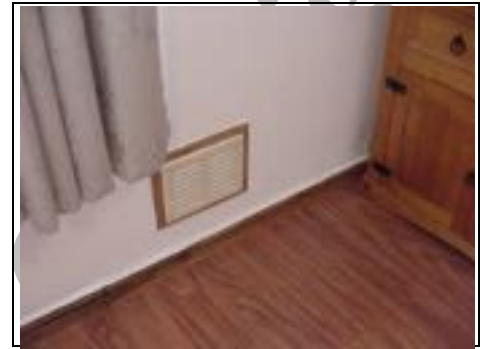
Vent in front room for fireplace
