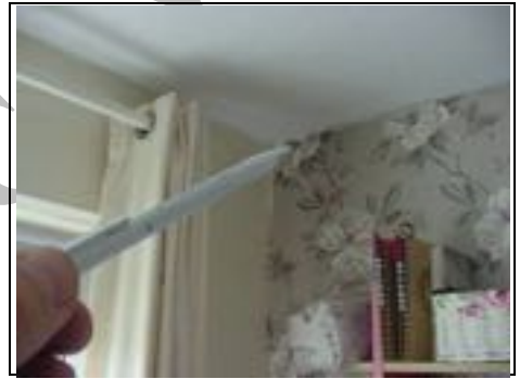
Black mould painted over in rear right bedroom
