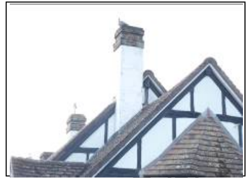
Cracks to render
