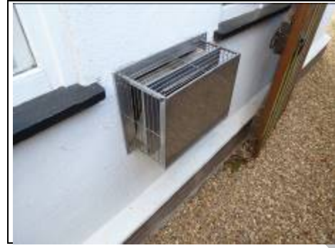
Flue from Worcester boiler
