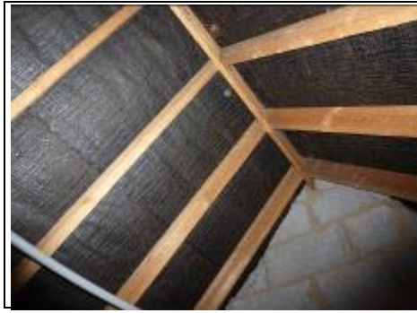
New left roof
