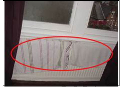
Drying washing on radiators can cause condensation
