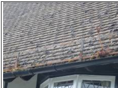
Tile guard rusting
