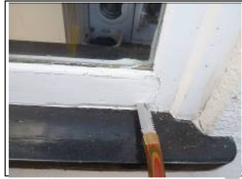
Rot to garage window
