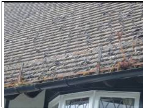
Tile guard rusting
