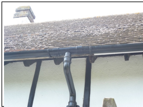
Exposed rafter feet
