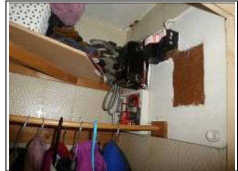
Old fuse board
