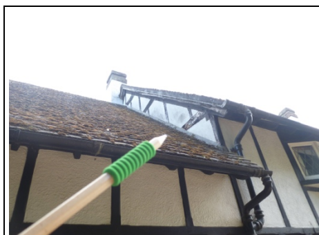
Rot to gable end
