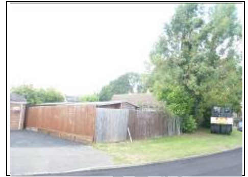
Rear left fence in poor condition
