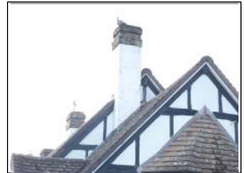
Cracks to render
