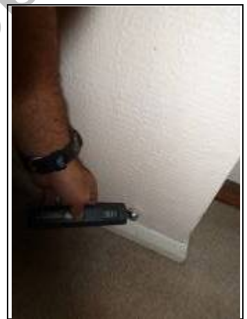
High damp meter reading
