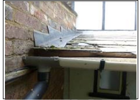
Tiles on end could be asbestos
