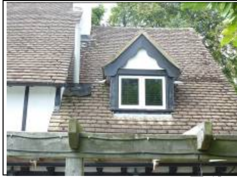
Deterioration to rear dormer
