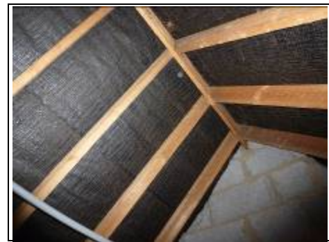
New left roof
