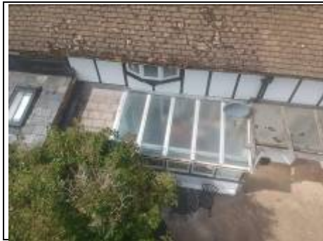
Georgian wire polished plate glass roof
