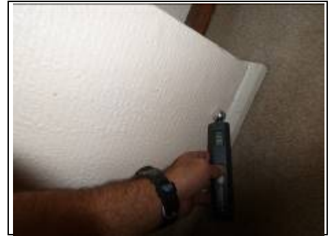
High damp meter reading
