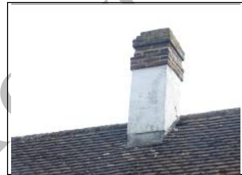
Crack to render of middle chimney
