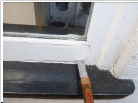
Rot to garage window
