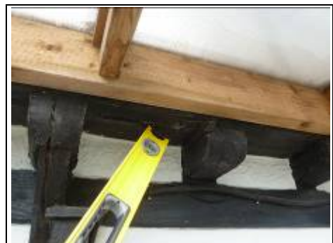
Rot starting to occur in jetty timbers to rear
