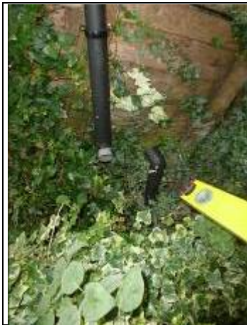
Downpipe to right loose
