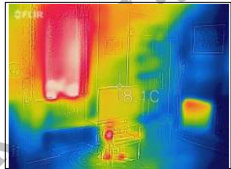
Heat coming in through window and warmth of the radiator, with the blue being the coldness of the walls (not your property)
