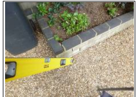
Small tree to front causing movement to dwarf wall
