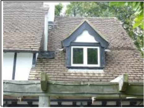
Deterioration to rear dormer
