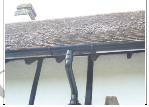
Exposed rafter feet
