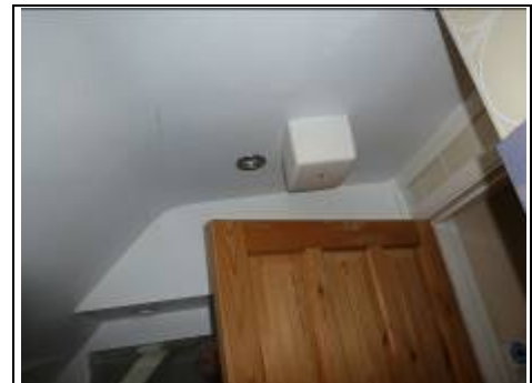
Extract fan in bathroom
