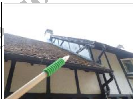
Rot to end timbers of gable end
