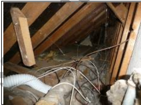
Extract trunking within roof space
