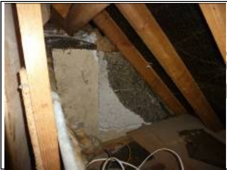
Right roof space – gable end of next doors property old style plaster
