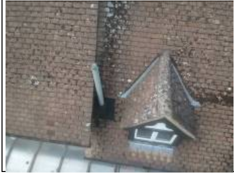
Soil and vent pipe
