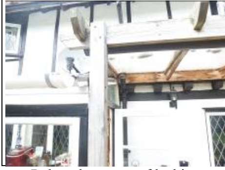
Polycarbonate roof leaking
