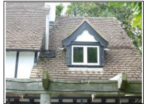
Deterioration to rear dormer
