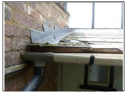
Tiles on end could be asbestos
