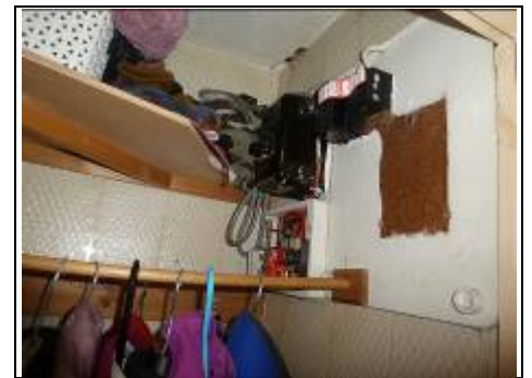
Old fuse board
