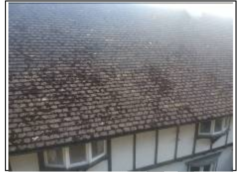
Moss on roof ~ Aerial View - 360 Photo ~
