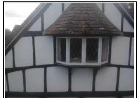
Oriel window deteriorating
