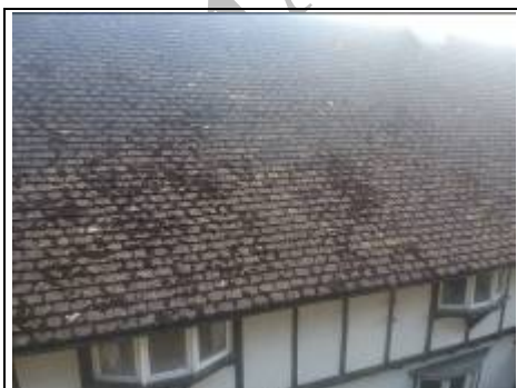
Moss on roof ~ Aerial View - 360 Photo ~
