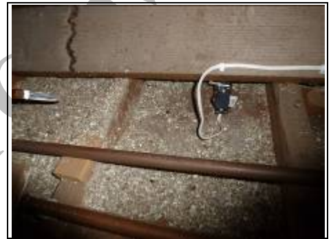
Lights not capped properly
