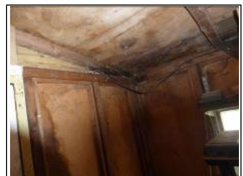
Dampness in shed
