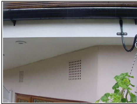
Crack at high level
