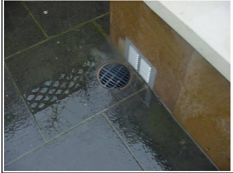
Airbricks acting as a gutter to the rear
