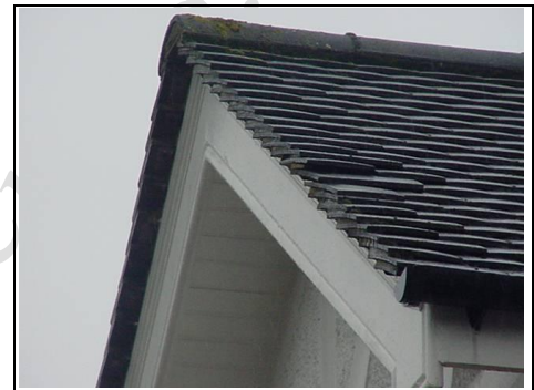
Tiles slightly displaced to the front
