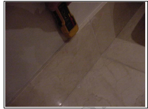
Low level rising damp
