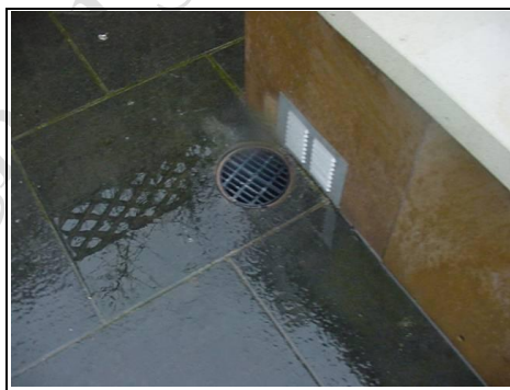
Airbrick acting as a gutter
