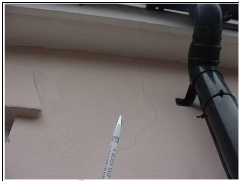
Cracking to the rear left hand side
