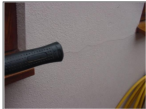
Cracking to the render
