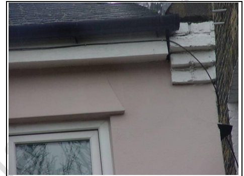
Drip details over the window on the render to the rear
