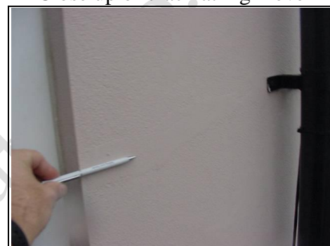
Old cracks that have been repaired previously
