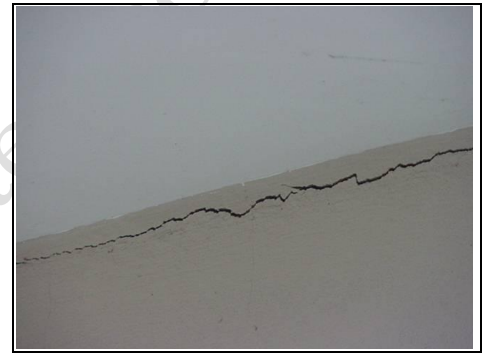
Close up of crack at high level
