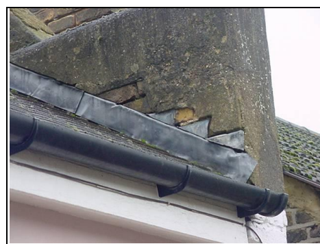
Poorly fitted flashing to the rear left hand parapet wall
