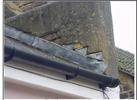
Poorly fitted flashing to the rear left hand parapet wall
