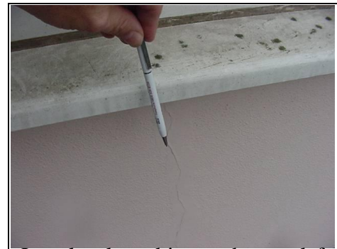
Low level cracking to the rear left hand side
