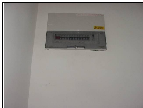
Fuse Board on first floor
