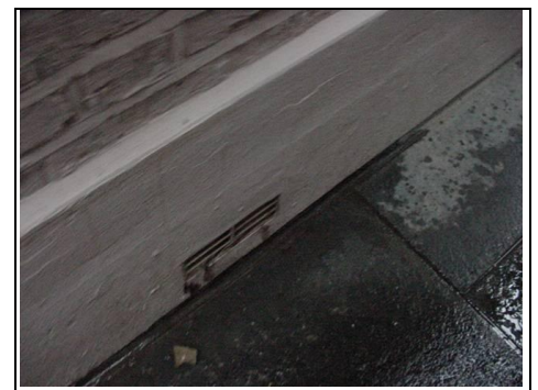
Airbrick acting as a gutter on the right hand side
