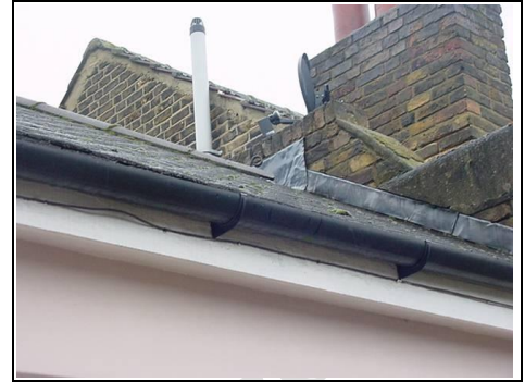
Soil and vent pipe
