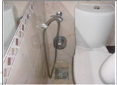
Washer unit in downstairs w.c. is leaking
