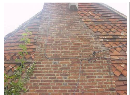
Chimney one – wrongly repointed in a cement mortar
