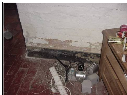
Lots of rising damp – paint coming off, we believe this to be a plastic based paint
