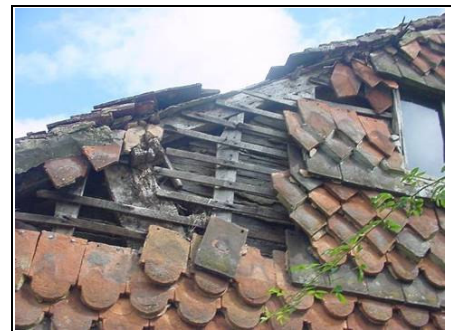
Vertical tiles coming off to left hand side of building
