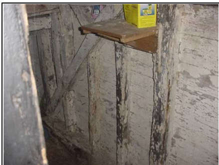
Lime washed timbers – this is how the timbers would have originally been
