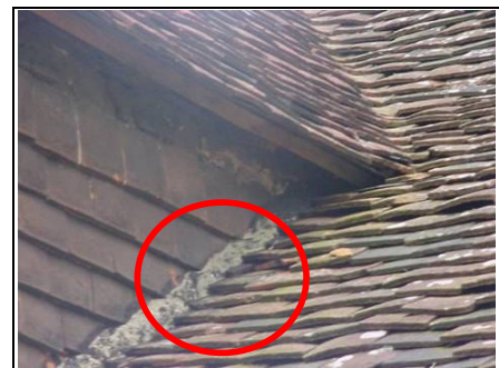
Cement flashings rather than lead flashings
