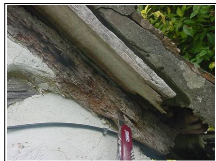
External timbers with woodworm which no longer looks to be active
