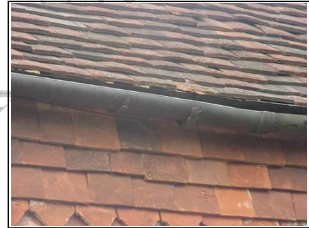
This gutter does not look to have a fascia board
