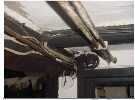
Surface mounted plumbing – plumbing could be better concealed
