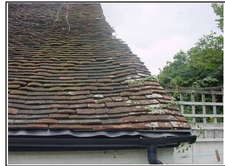
Protective underlayer poking out from underneath the tiles.
