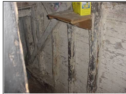
Lime washed timbers – this is how the timbers would have originally been
