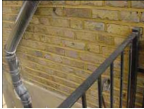
Modern cement re-pointing to wall
