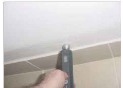
Damp reading at skirting
