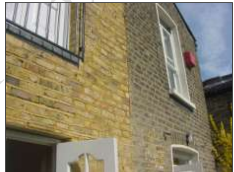
Bulge in brickwork to the rear
