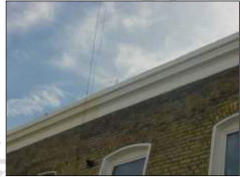
Future roof problems, we could see vegetation growing above the side of the parapet walls
