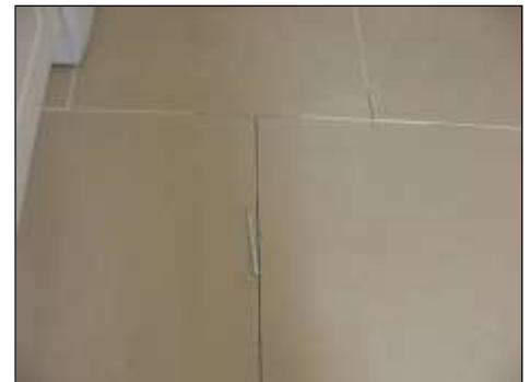
Tiles in kitchen laid without expansion joints, a hard tile surface onto a moving timber surface
