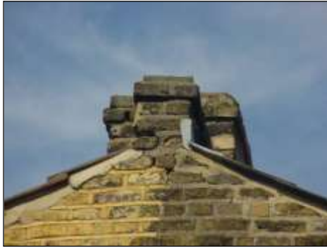
Rear chimney viewed from ground level, (the only chimney we could see).
