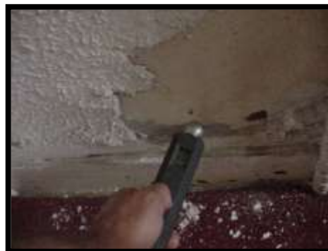
High damp meter readings in the hallway
