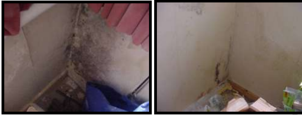
Mould to the corners of the bedroom
