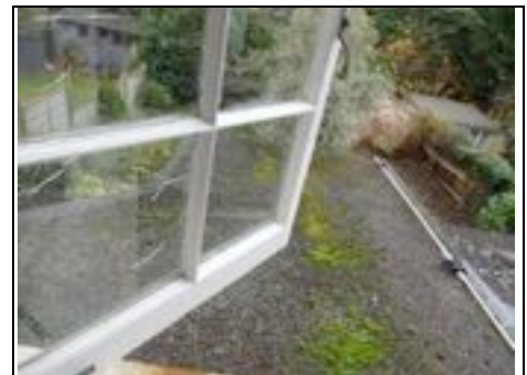
Broken window, moss on roof and condensing pipe from boiler
