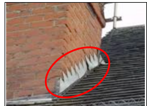
Flashing coming away
