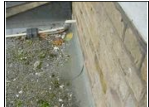
Felt flashing, we prefer a lead flashing
