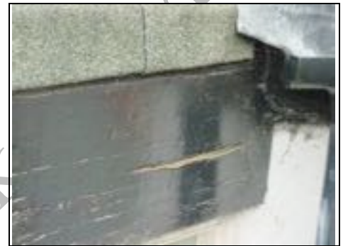
Fascia board needs redecorating
