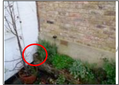
Planter bed to rear left side, maybe causing dampness internally
