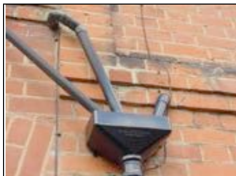
Next door's hopper head overflowing
