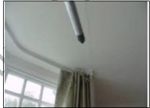
Crack in ceiling to bay window
