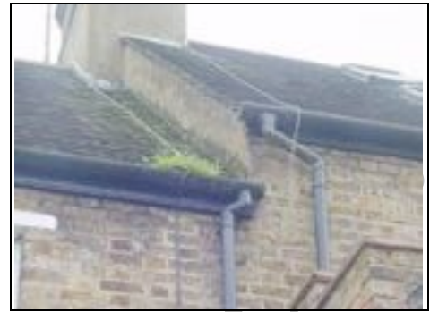
Grass growing from gutter
