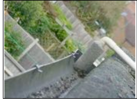
Condensing pipe going into downpipe. We have known there to be problems with these freezing as it's a condensing pipe from a boiler
