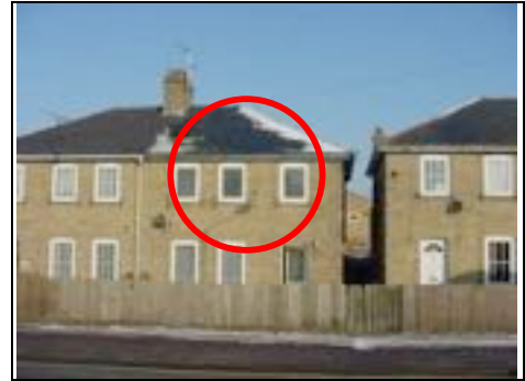
Inappropriate double glazed windows change the look of the property Red circle is insulated roof indicated as snow is not visible
