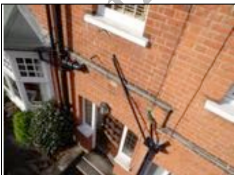
Soil and vent pipe and next door's hopper head Aerial view – 360 photo
