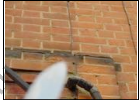
Soft red brickwork spalling
