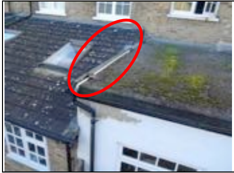
Condensing pipe from boiler Aerial view – 360 photo
