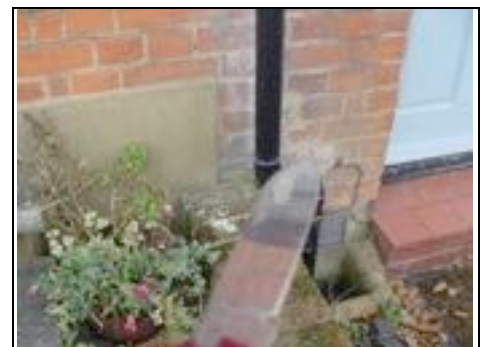
Dampness may get into your property from the overflowing hopper head
