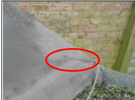
Splits in asphalt
