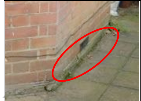
DPC to next door property
