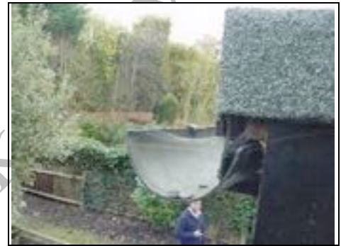
Missing end cap (and next door neighbour!)
