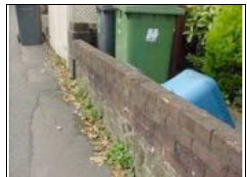
Crack to front wall
