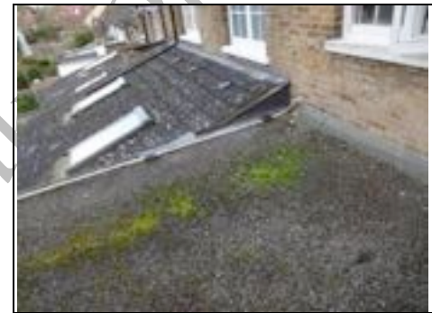
Moss on rear left flat roof Aerial view – 360 photo
