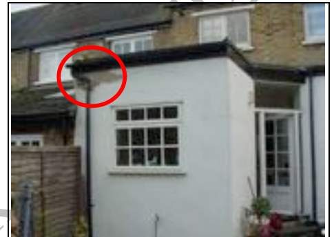
Painted render to rear extension with unpainted area around gutter
