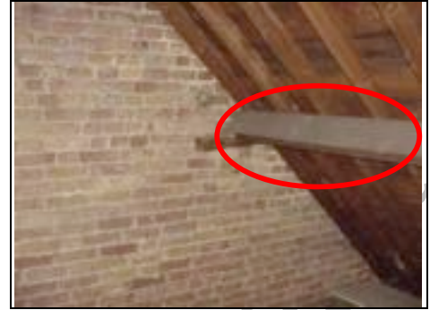
Purlins need periodic inspection
