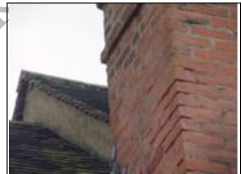
Brickwork needs repointing to rear right chimney
