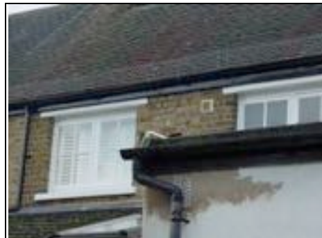
High level air vent in rear extension
