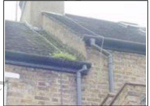
Grass growing out of rear gutter
