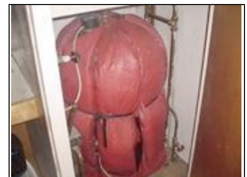
Older style cylinder with loose insulation jacket
