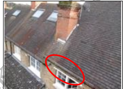
Displaced tiles. Tile guard at bottom Aerial view – 360 photo
