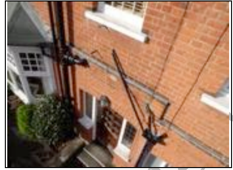
Soil and vent pipe discharging into next door's hopper head
