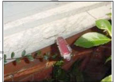
Minor wet rot in timber window frames
