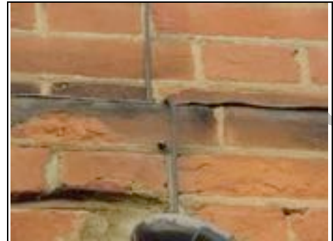
Close up of cement mortar and spalling brickwork
