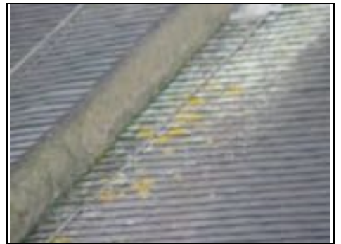
Step in roof
