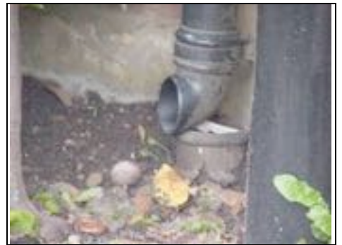
Downpipe discharges onto ground, which could cause dampness
