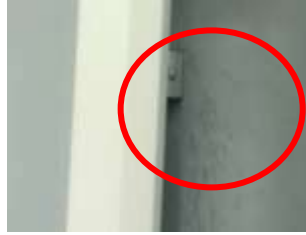
Downpipe with water damage to metal backing
