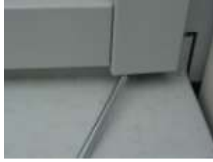
Cut metal around window which will rust
