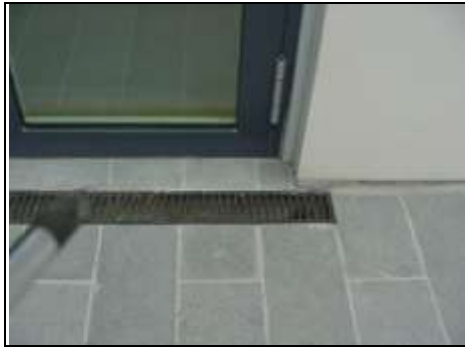
Threshold on left side has running gulley
