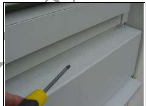
Weathering of windows
