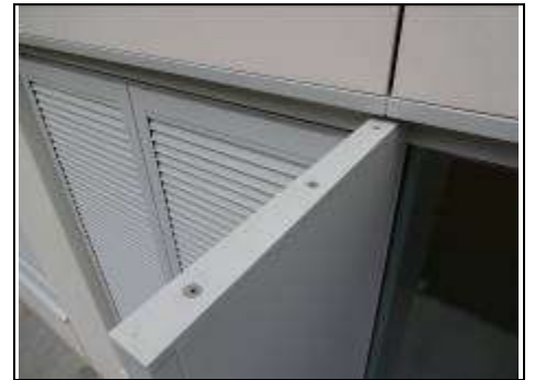
Rust to top of shutters. A flat surface like this will promote rust relatively quickly if not painted properly.
