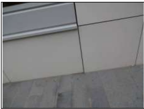
Rain cladding not sealed properly to ground in all areas
