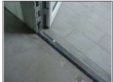
Right side has no running gully and is same level inside and outside
