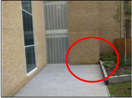
High ground level against brickwork
