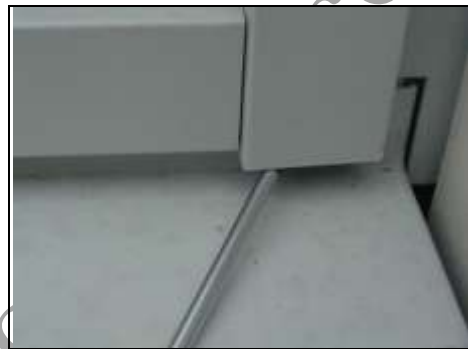
Cut metal around windows which will rust
