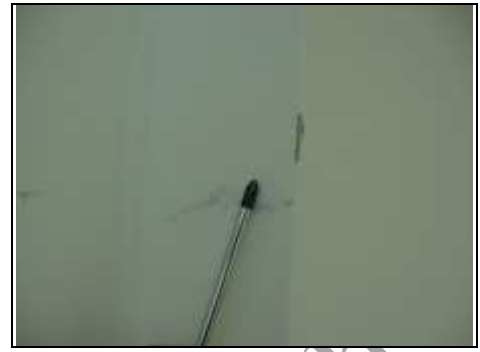
Wall marked in Room One
