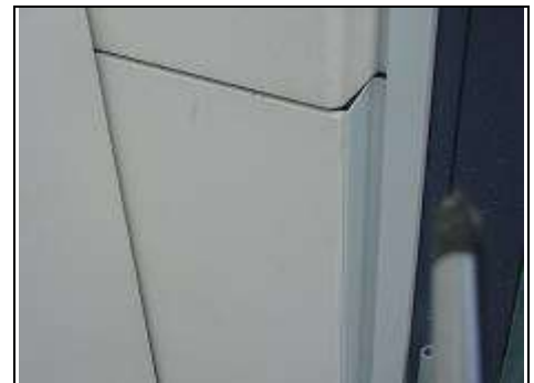
Poor detail around left double doors
