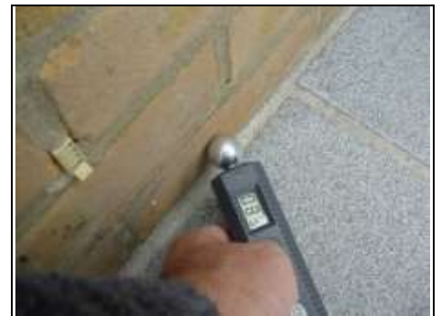
Dampness present on brick wall
