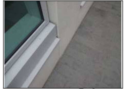
Where does water drain to
