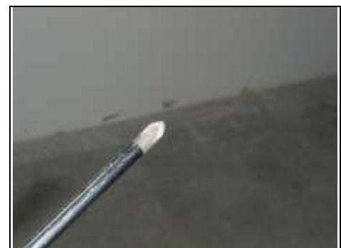
Wall marked at base in open plan room right
