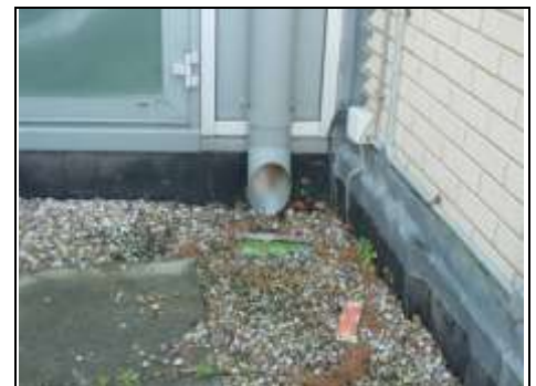
Rainwater pipe discharging onto inverted roof with no obvious flow path
