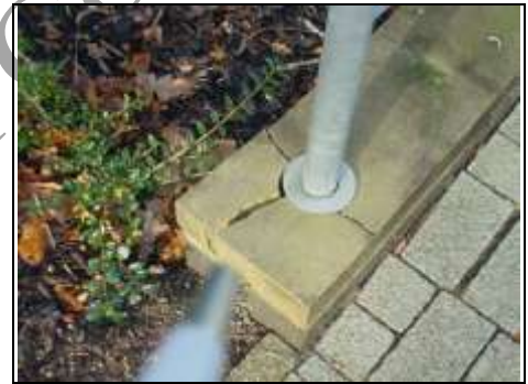
Damage to ramp access
