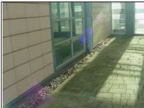
Moss to paved area at front
