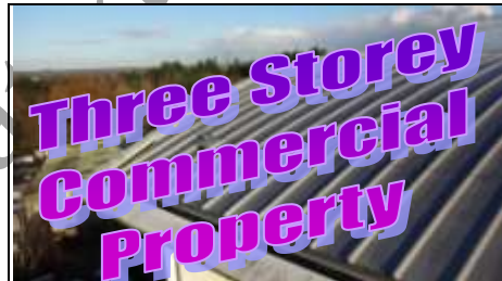
Discoloring to corner indicating water damage
