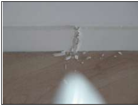
Dampness in skirting of restaurant
