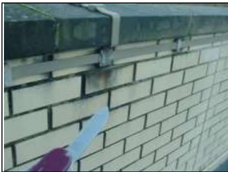
Example of coping stones joints leaking
