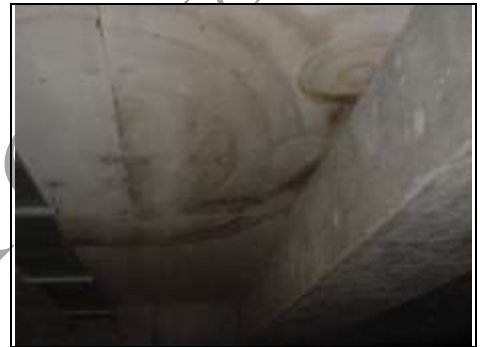
Staining to concrete
