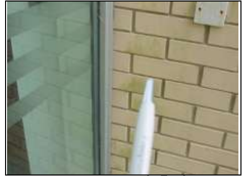
Moss impregnated into brickwork
