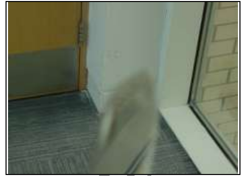
Dampness in first floor corridor from leaking hopperhead
