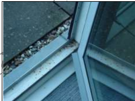
Rust spots to door
