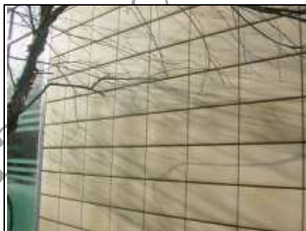
Moss and lichens to rain cladding on left gable end
