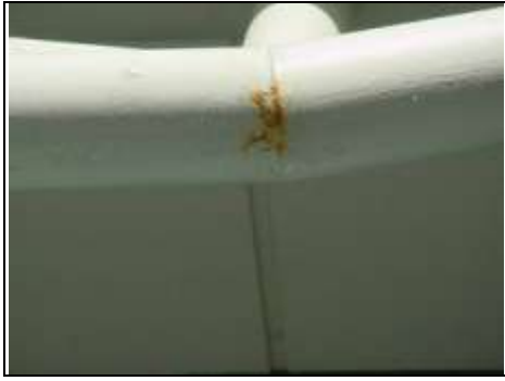
Rusting to tubular steel
