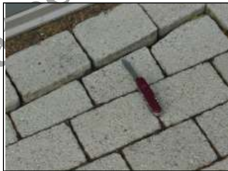
Unevenness in external cobbles
