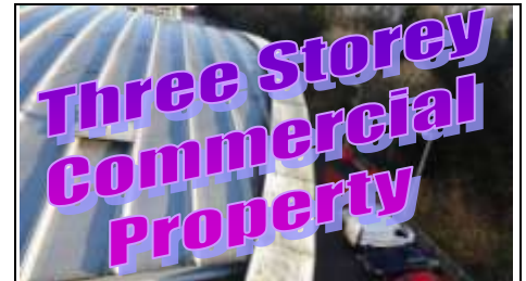
Ends of roofing panels coming away
