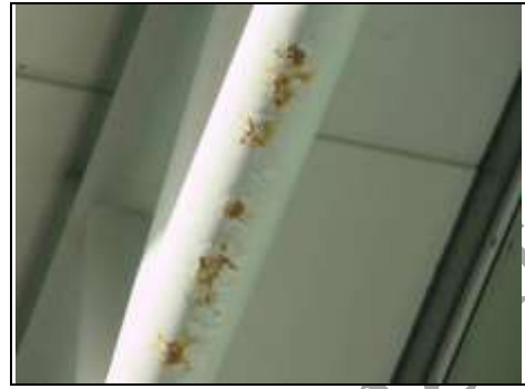
Rusting to tubular metal frame
