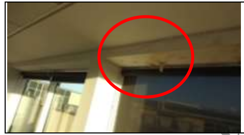
Leaks coming into property from flat roof
