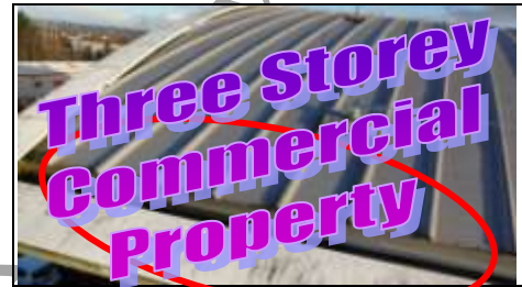
Deterioration to end of sheets of domed roof on front left
