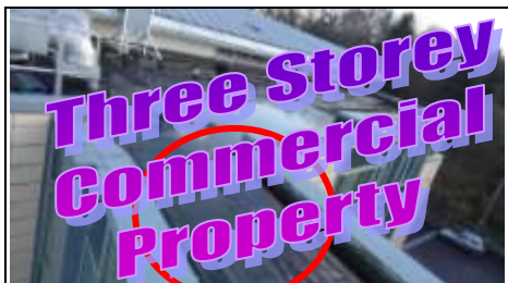
Rucking and ponding on mono-ply roof
