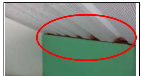
Marks where roof meets wall looks to be expanded foam
