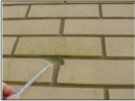
Damage to brickwork
