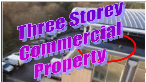
Metal coping over rain cladding with water sitting on it
