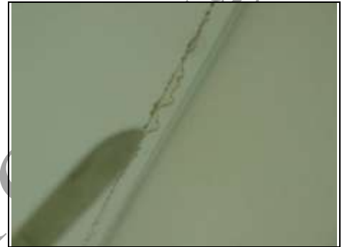
Cracking to ceiling ground floor front right
