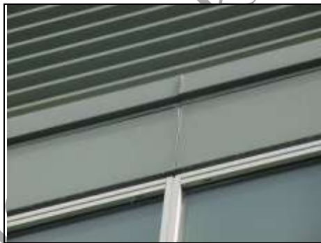
Weathering to joint
