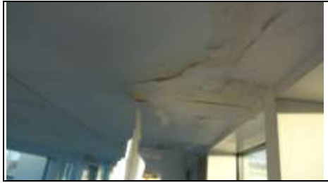
Leaks in corridor under flat roof
