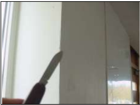
Dampness in restaurant
