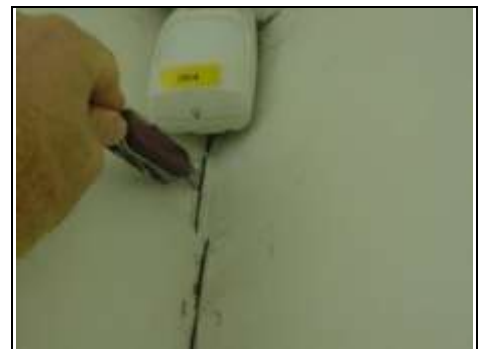
Cracking to wall ground floor front right
