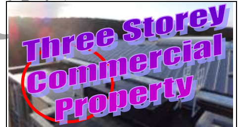
Ponding to right flat roof
