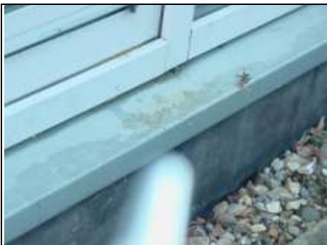
Rust to sill
