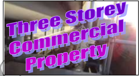
Rainwater from left domed roof discharging onto flat roof with nowhere to go as far as we could see
