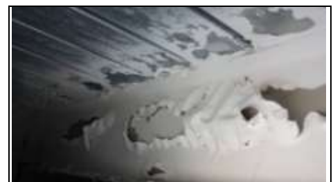
Paint perishing on top floor
