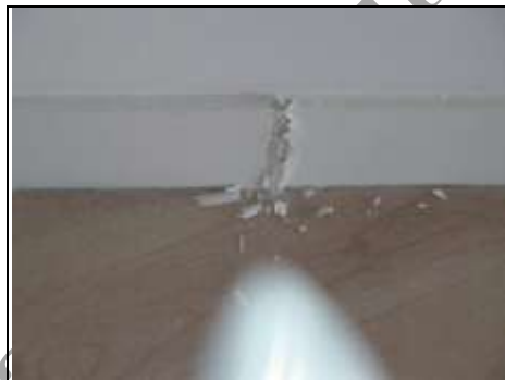
Dampness in skirting of restaurant
