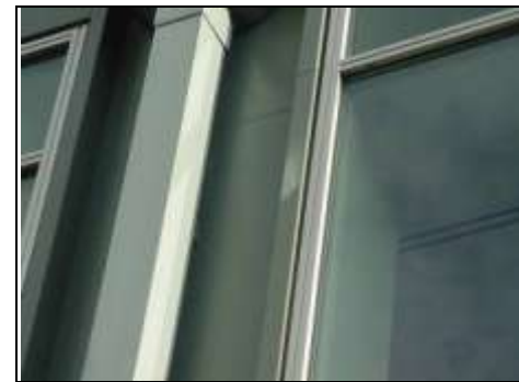
Weathering to metal or it has been resprayed and missed an area
