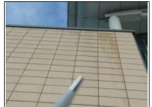
Rainwater going down rain cladding from coping above
