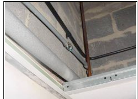
Copper and plastic piping leaking
