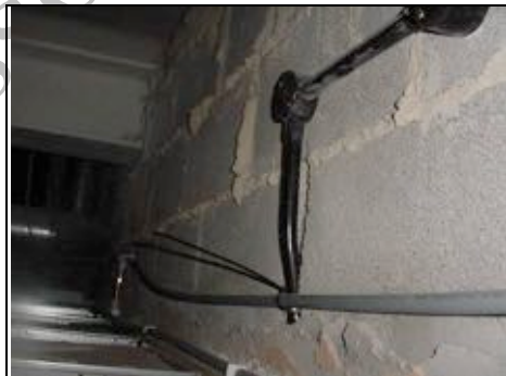
Copper and plastic piping leaking
