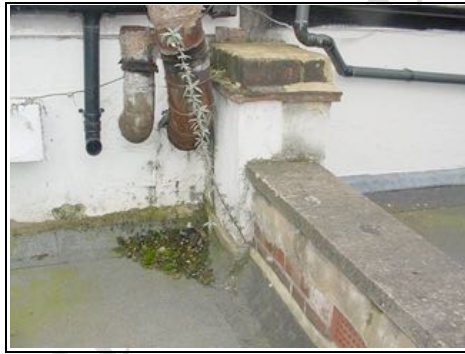
Junction of toilet roof and roof over the shop. Water is discharging onto render which is part of the reason causing dampness below
