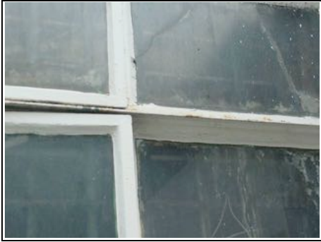
Window not shutting
