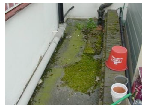
Close up of rear flat roof over the shop with moss and signs of leak below
