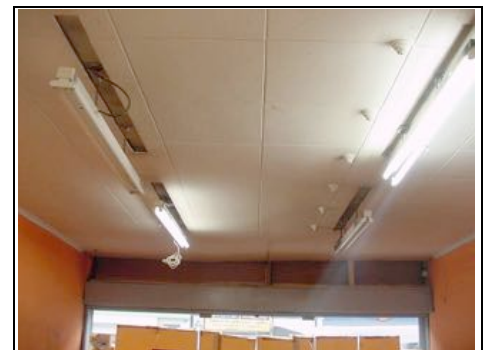
Ceiling is water damaged 15
