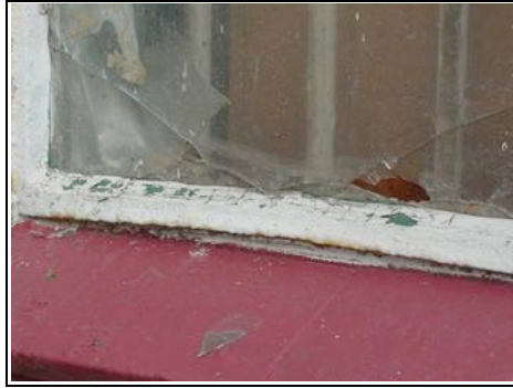
Broken glass in toilet window
