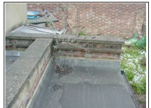
Roof over toilet with tree growing out of parapet wall
