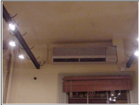
Heaters over windows
