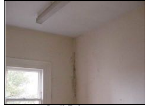
Black mould to corner
