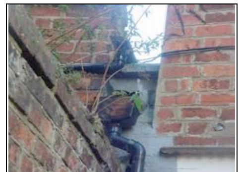
Rusting cast iron hopper head
