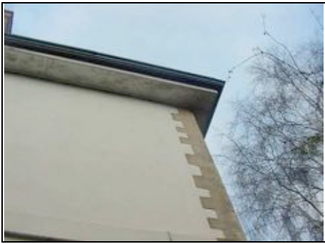
Fascias and soffits deteriorating
