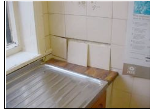
Tiles off wall
