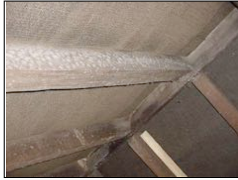
Mould due to lack of ventilation
