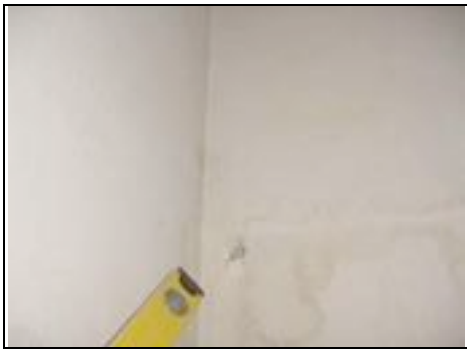
Dampness coming through
