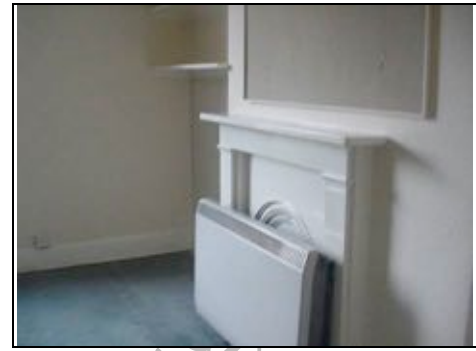
Electric fire in front of fireplace
