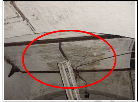
Dampness within basement causing rust to cast iron
