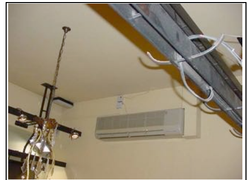
High level heaters
