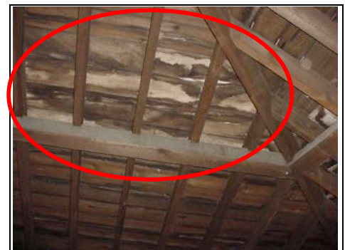
Dampness coming through close boarding
