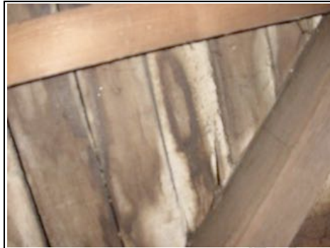
Signs of dampness to boarding
