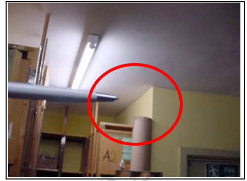
Cracks between studwork partitions and ceilings
