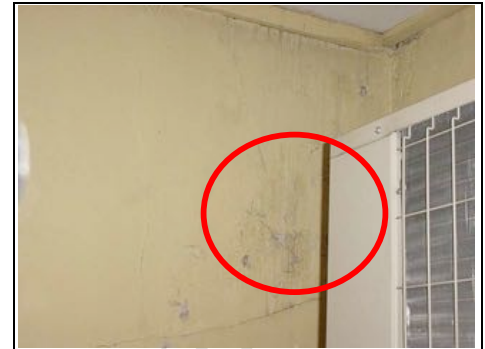
Dampness in plant room
