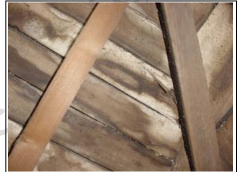
Dampness to boarding
