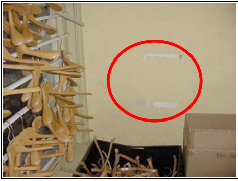
Heavily marked wall in store room
