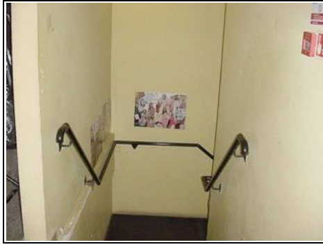
Staff room staircase marked walls and old pictures
