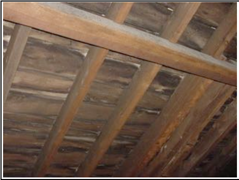
Dampness coming through the roof
