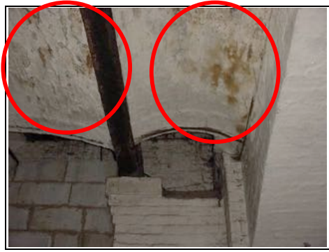
Dampness to Vaulted brickwork coming through from ground floor
