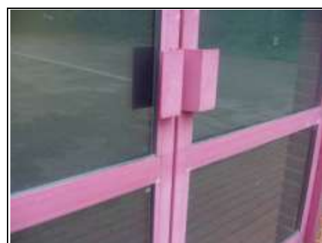
Fading paintwork to metal windows
