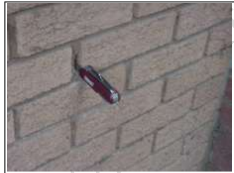
Some of the perpendicular ends have not been butted up
