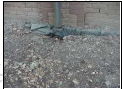
Downpipe no longer connected and seems to be blocked
