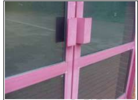
Front door paintwork fading
