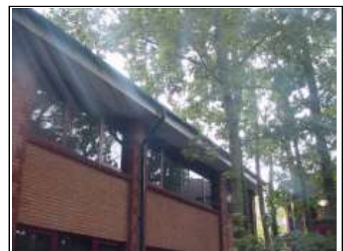
Trees close to building
