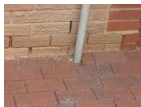
Weathering to the bricks and joints, we would recommend a French drain is added
