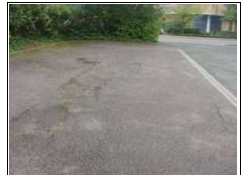
Car park unmarked and deteriorating
