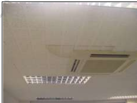
Staining to first floor rectangular ceiling grid system
