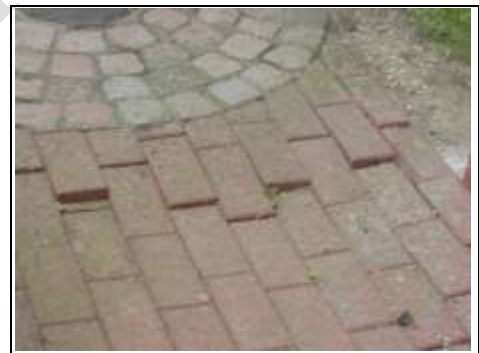
Settlement in brick paves at front of property
