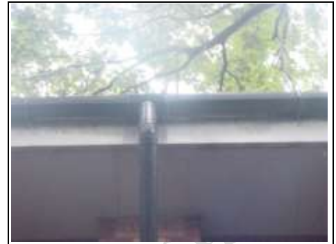
Close up of rear gutter and downpipe, staining to fascia board which indicates leaks. Note the tree hanging directly over this guttering
