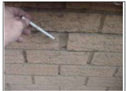
Raking crack to rear brickwork
