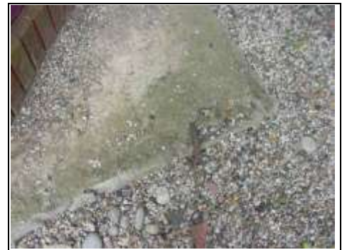
Reinforcement visible on neighbouring property indicates poor standard of workmanship
