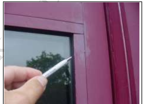
Close up of front door paintwork fading
