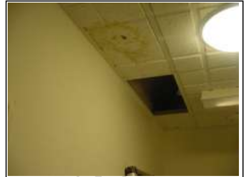
Signs of water leaks in ceiling system
