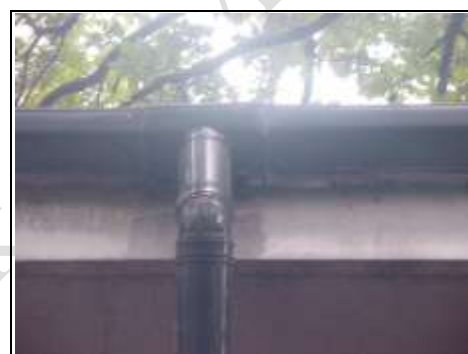
Fascia board stained due to leaking gutter and downpipe
