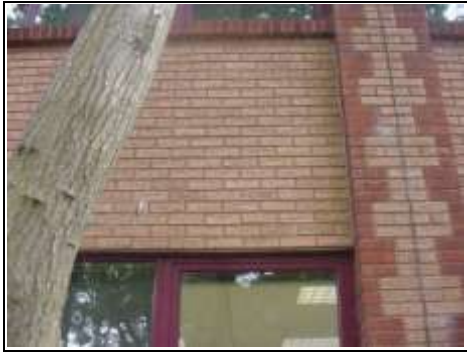
Brick panelling around column to right hand side, expansion joint and left brickwork panel close to tree
