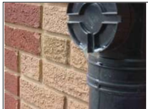
Residue discharging from front downpipe which we can only assume is from leaves and other debris in the gutters
