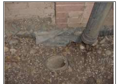
Rear downpipe not connected
