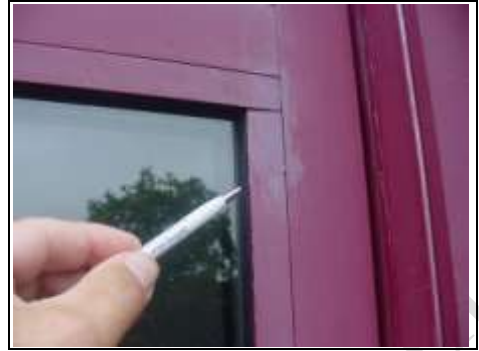
Deteriorating paintwork to metal window
