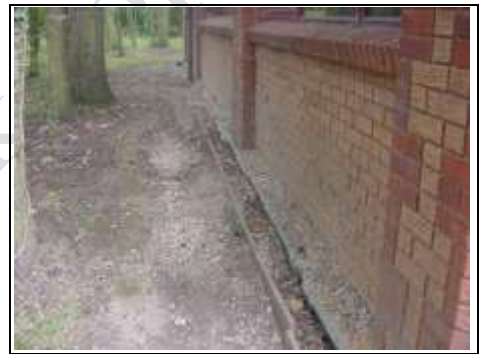
Settlement to rear possible old French drain
