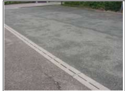
Unsuitable drainage to car park
