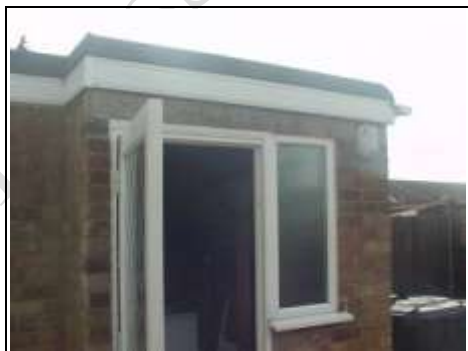
Example of a concrete lintel – can you notice where the cold bridging would be in this photo?
