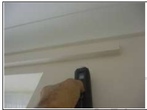
Dampness and condensation around the concrete window lintel
