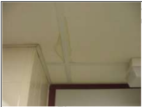
Staining to ceiling leaking from above
