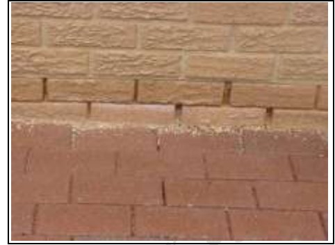
Mortar weathered away
