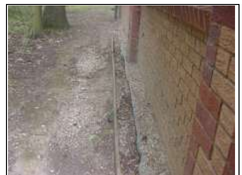
Ground adjacent to rear downpipe sinking
