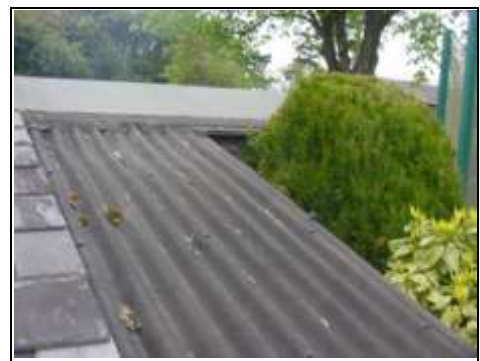
Fibre roof, also to the rear, we would replace with a slate roof in keeping with the rest of the property
