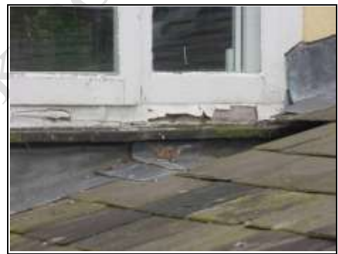
Timber window degrading
