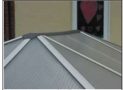
Poor quality repair to the ridge in Flashband that needs replacing
