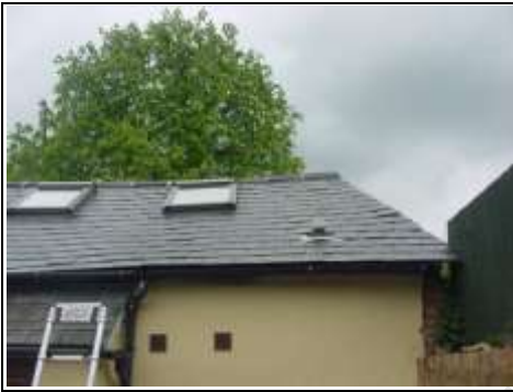
Undulation to rear building roof
