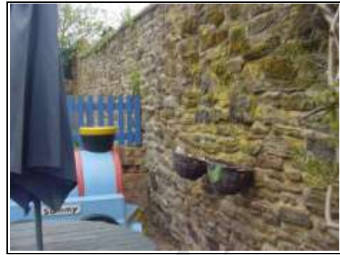
Bulging Boundary wall
