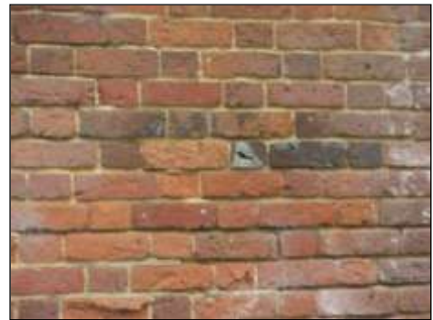
Brickwork in need of re-pointing
