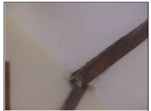
Tingles holding slates in place
