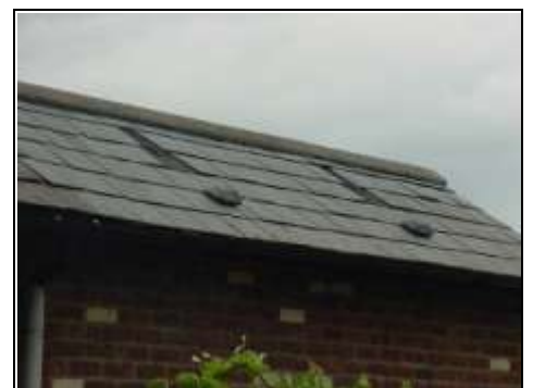
Rear of roof with missing slates
