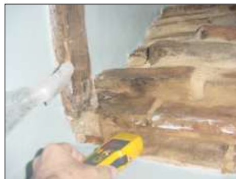
Dampness coming in from chimney one
