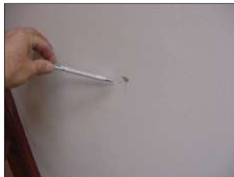
Plasterboard ceiling top floor degrading
