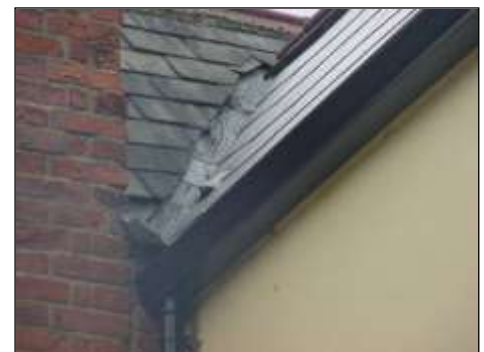
Natural slate to the left hand side and manmade slate to the right hand side and a lead valley gutter that has been tarred indicating that it has leaked
