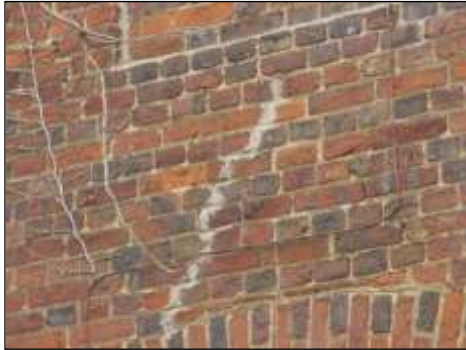
Cracking we believe this relates to gable end movement
