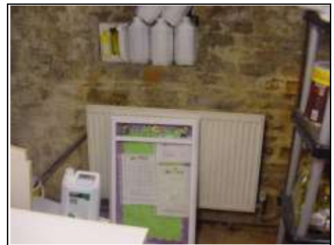
Radiator in the cellar
