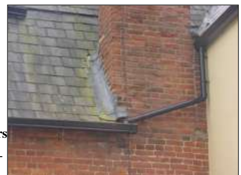
Unusual downpipe detail
