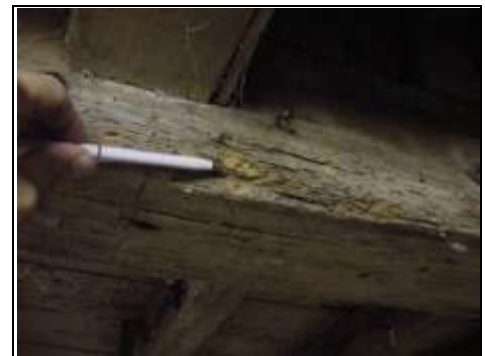
Signs of woodworm in basement
