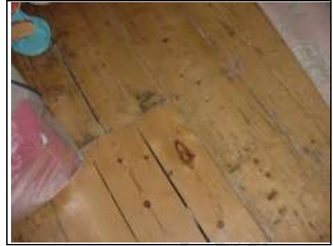
Top Floor: Older timbers have woodworm and there are new replacement timbers
