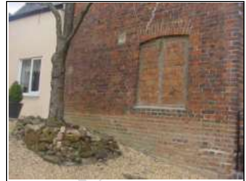
Incorrect cement mortar used to the base of the left hand side of the property for example
