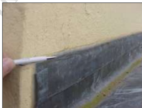
Mastic seal to the lead flashing indicating problems
