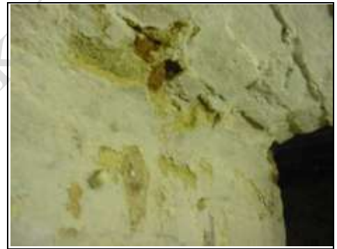
Spalling to chimney
