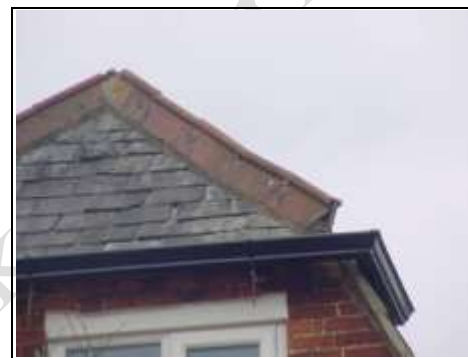
Guttering hiding fascias and soffits
