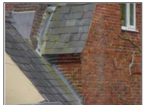
Lead tingles to left hand side of the roof and displaced slates to the right hand side
