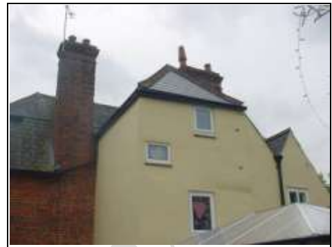
Repair work required to render
