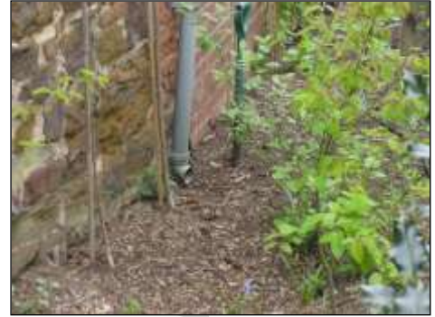
Rainwater discharges directly to the base of the property
