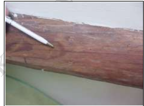
Signs of woodworm in rear building
