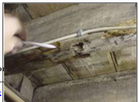
Signs of woodworm in basement
