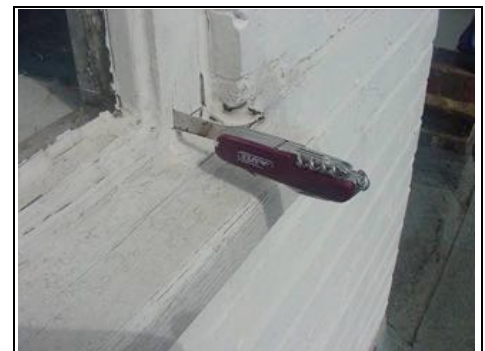
Rotten timber window at the rear of the property
