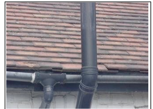
Gutter needs repairing again has previously been repaired
