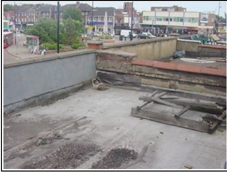
Leak on corner
