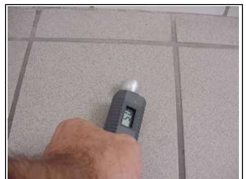
Damp readings taken within the Staff toilets
