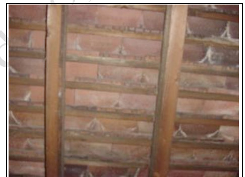
No protective underlayer
