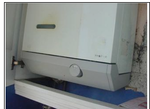
Potterton Profile boiler in kitchen
