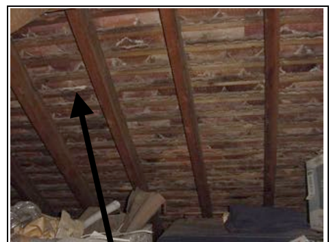
Efflorescence to underside of roof tiles
