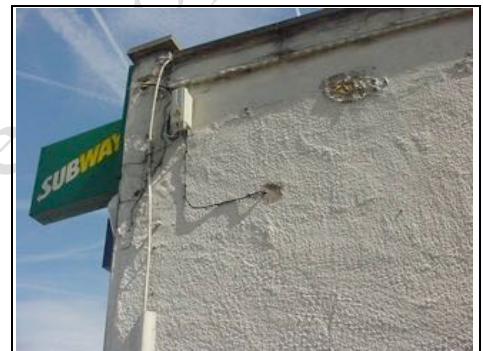
Spalling to render on the right hand side caused by the leak from the roof
