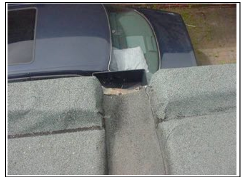
Box gutter to left hand side of rear flat roof blocked
