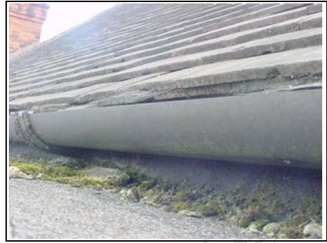
Flat roof over bay window at the front of the property leaking
