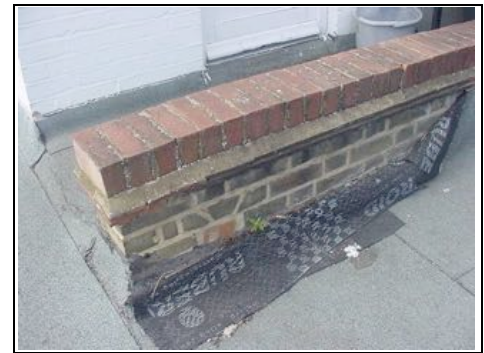
Felt flashing coming away
