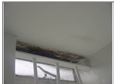
Black mould in Staff toilets
