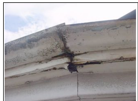
Leaking and rusting gutters
