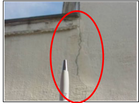
Crack between single storey extension and the main building
