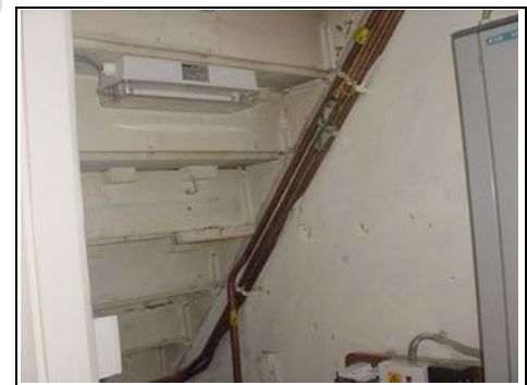
Stairs not lined
