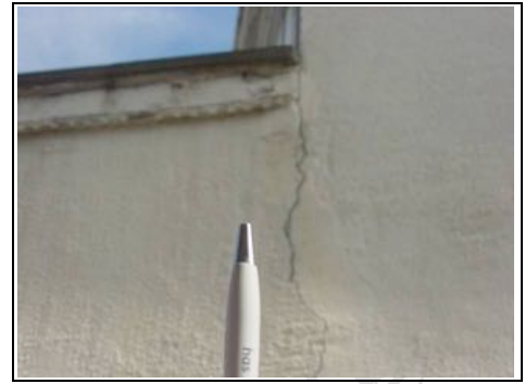
Cracking to the render on the right hand side
