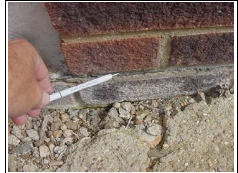
The damp proof course is too low
