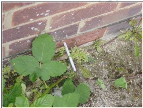
Airbrick broken and too low
