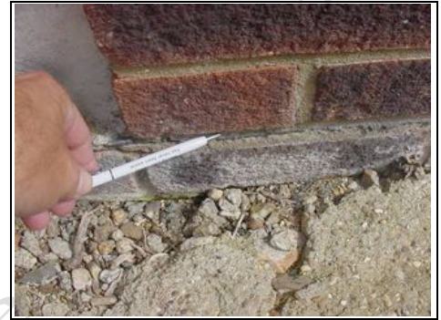
Damp proof course too low
