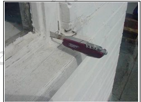
Knife test reveals deterioration to timber windows
