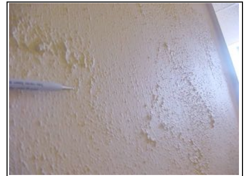
Artex/asbestos on walls
