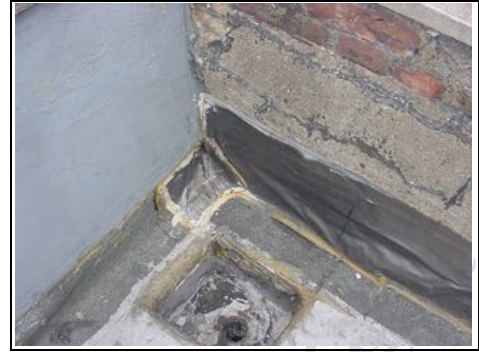
Previous Flashband repair to corner
