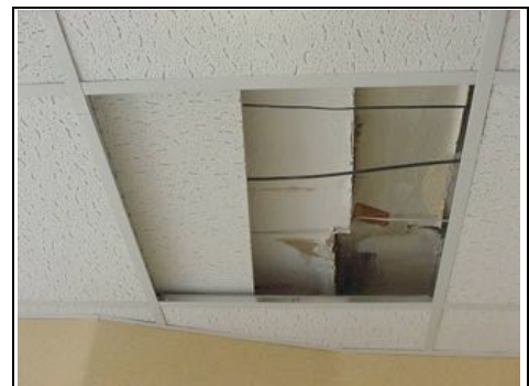
Decking to ceiling in retail unit front of house coming away
