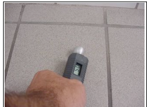
Damp readings indicating dampness in Staff toilets on ground floor
