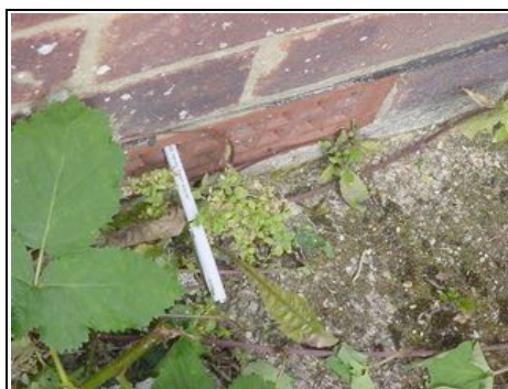
Close up of airbrick which is too low
