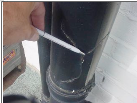
Soil and vent pipe cracked
