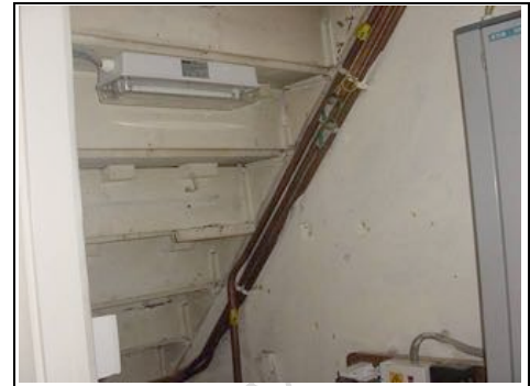
Stairs not lined
