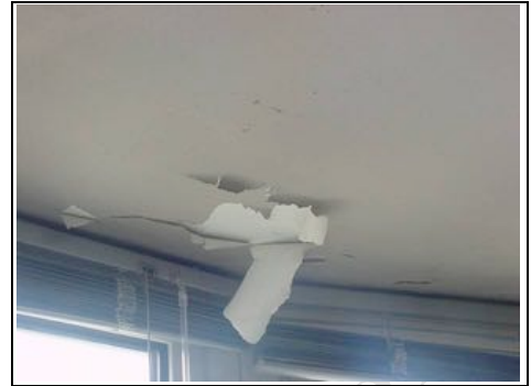
Flaking paint to bay window
