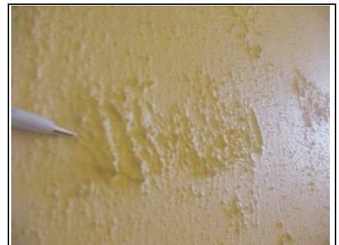
Artex/asbestos on walls
