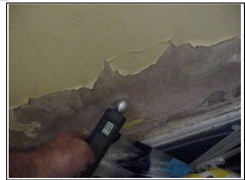
Dampness in private living accommodation showing readings of 101, typically we would expect to find 30-60
