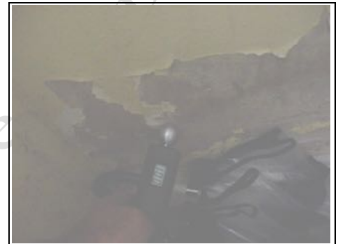
Testing for lateral dampness with readings over 100
