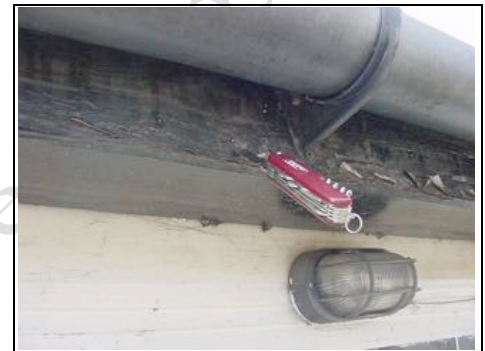
Fascias in a poor condition
