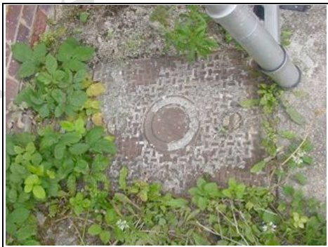
Unable to lift manhole at rear
