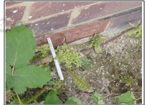
Air brick too low
