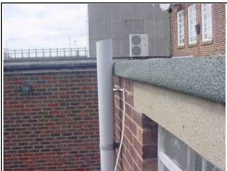
Soil and vent pipe not as high as it should be
