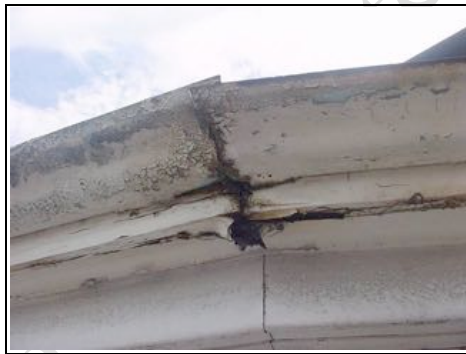
Front flat roof has a rusting cast Ogee gutter
