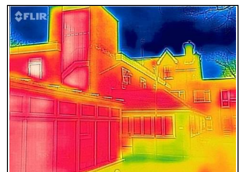
Heat coming through glazing to rear left side
