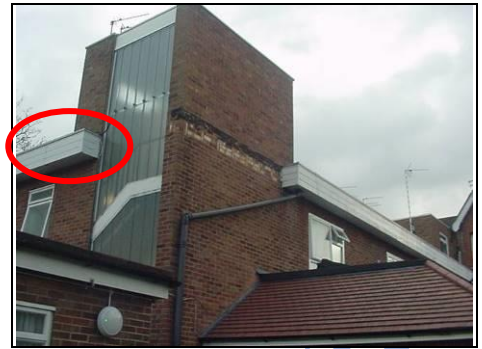
Dampness coming in this area
