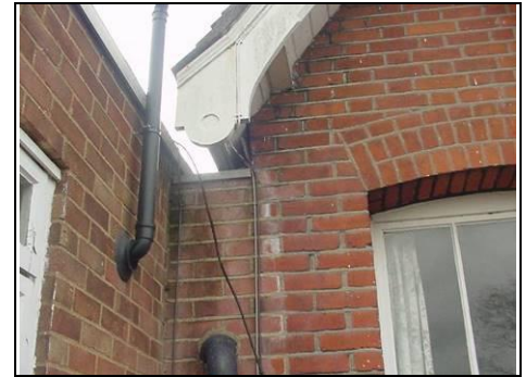
Second hidden box gutter to main roof overflowing
