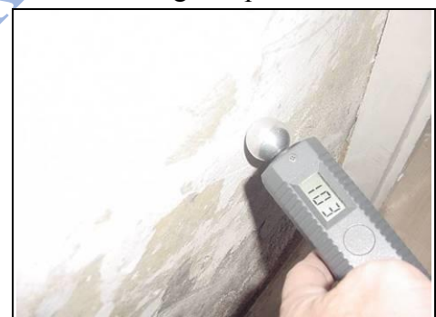
High readings of rising damp in basement
