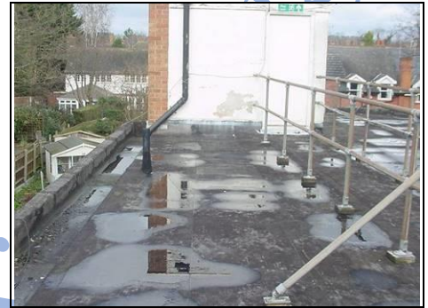
Ponding on two storey flat roof looking towards the lift
