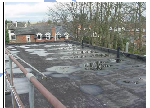
Ponding on two store left flat roof Aerial view – 360 photo
