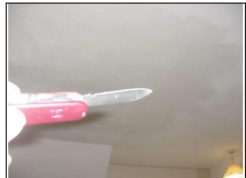
Repainting on ceiling. We assume this relates to water coming through
