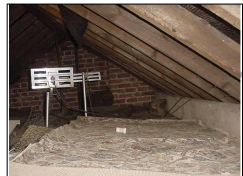
General view of right side of rear roof with mass of insulation
