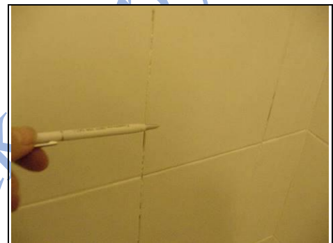
Weathering to tiles in en-suite
