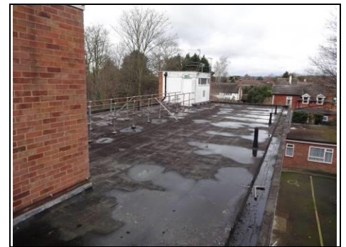
Roof of two storey extension looking towards lift tower Aerial view – 360 photo
