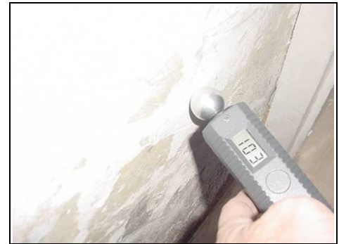
High damp readings in basement
