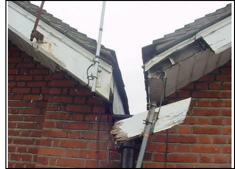
Broken aerials pulling fascia away
