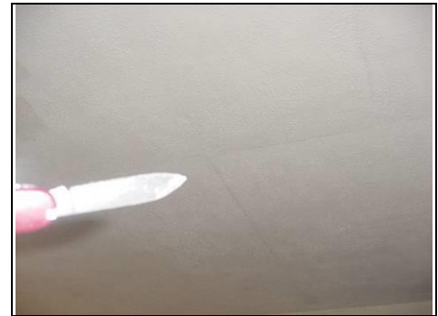
Textured paint may contain asbestos
