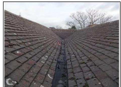
Close up of hidden valley gutter on main roof below box gutter Aerial view – 360 photo
