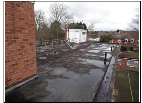
Ponding on two store left flat roof Aerial view – 360 photo
