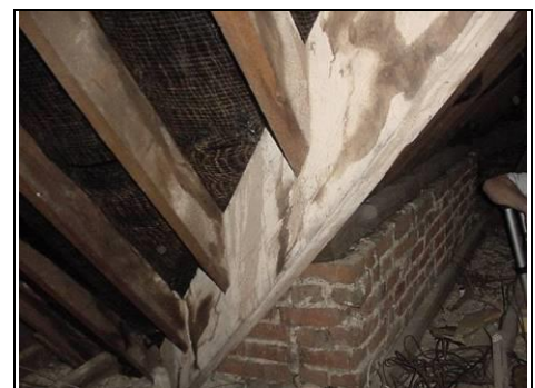
Dampness coming into valley gutter at front of property
