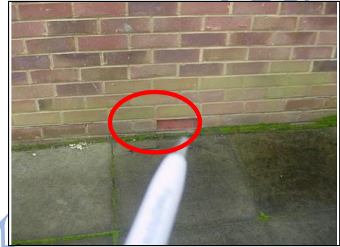
Airbricks acting as gutters
