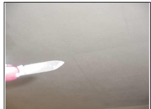
Textured paint may contain asbestos
