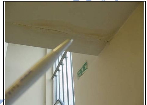
Damage in lift area likely to be caused by flat roof and deteriorating fascias and soffits
