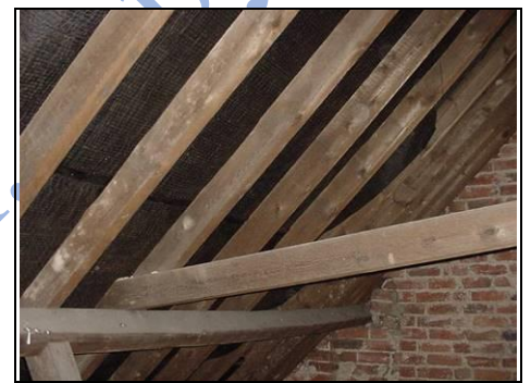
This photo shows common rafters in the front roof (the ones that form the pitch of the roof), the dark area between is the underlayer
