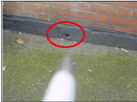
Air brick over basement needs clearing
