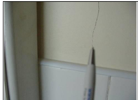
Hairline cracking, possibly from roof above
