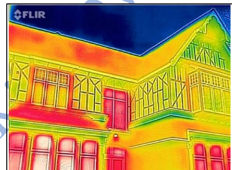
Thermal imaging of the front the property. Red areas indicating heat loss areas
