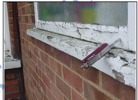
Rotten timber to accommodation area on top floor
