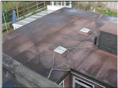
Left side of roof showing weathering of mineral felt Aerial view – 360 photo
