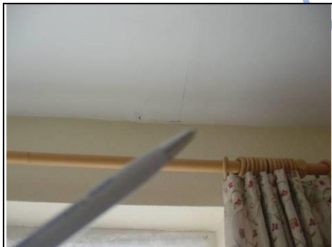
Leak coming in from flat roof above
