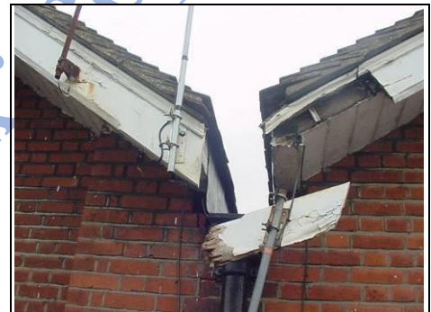
Broken aerials pulling fascia away
