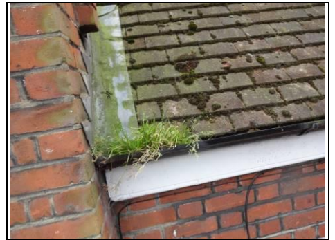
Grass growing out of gutter Aerial view – 360 photo
