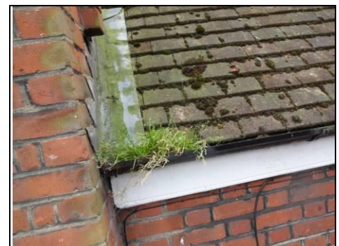
Blocked gutters Aerial view – 360 photos
