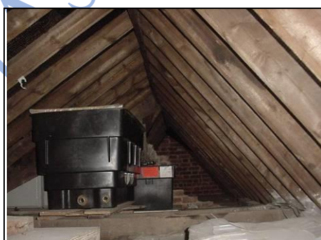
Water tanks in the front roof
