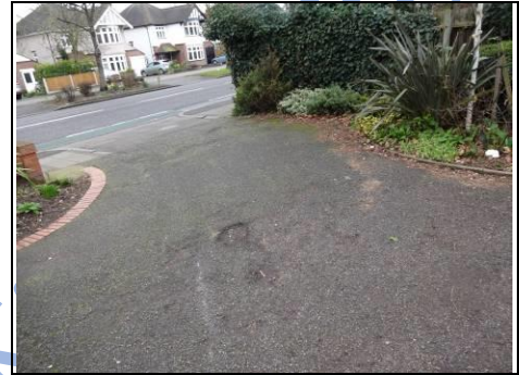
Deterioration to car park
