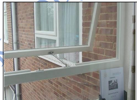
Window needs a restrainer adding to it
