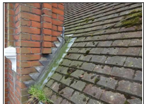
Trap behind front right chimney which is catching vegetation Aerial view – 360 photo
