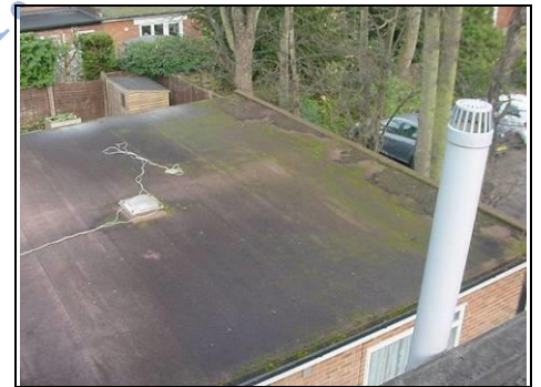
Leaves and moss on right side of roof Aerial view – 360 photo
