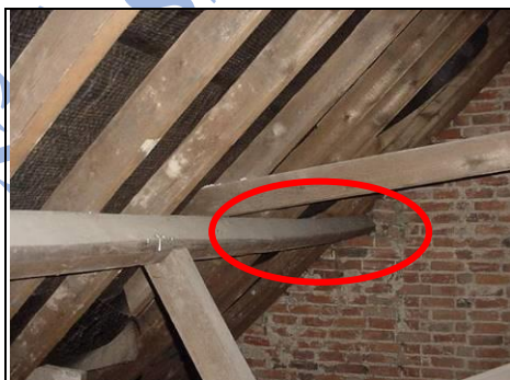
Deflection to purlin in front roof
