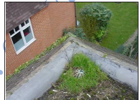
Blocked gutter on flat roof to left side
