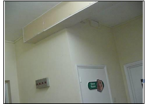
Unfinished plasterboard that looks to be from a waste pipe
