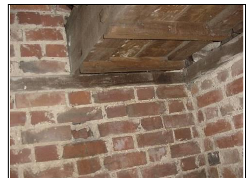
Under side of box gutter visibly leaking within main roof space
