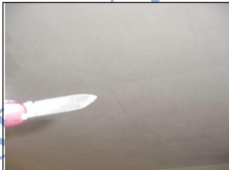
Hairline cracking and textured paint on ceiling in top floor accommodation
