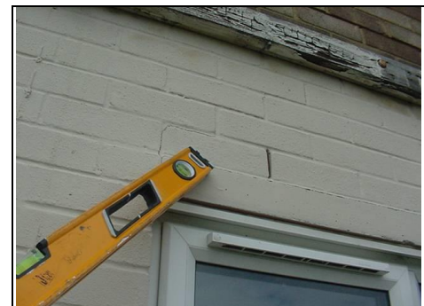
Cracking to rear right
