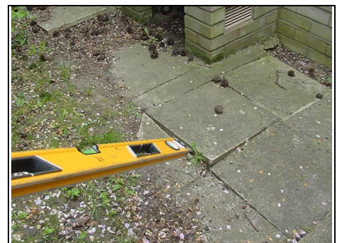
Trip hazard on footpath
