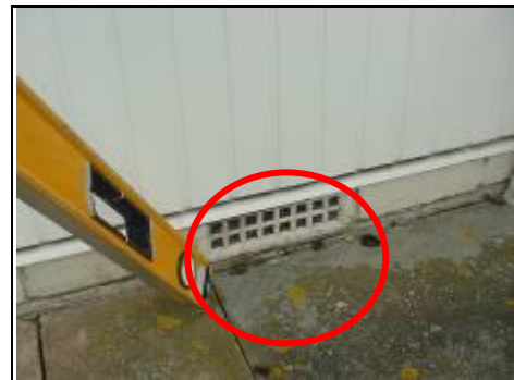
Airbrick acting as gutter
