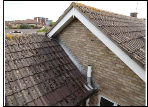
Soil and vent pipe
