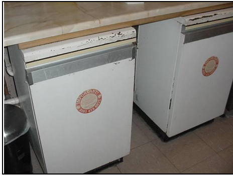
Boilers in kitchen
