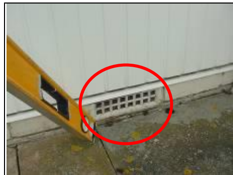
Airbrick acting as gutter
