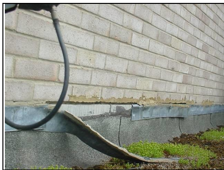
Lead falling off
