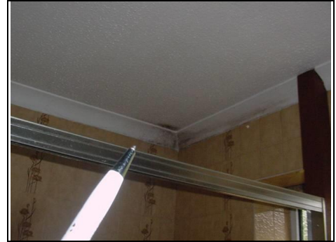
Mould in first floor bathroom
