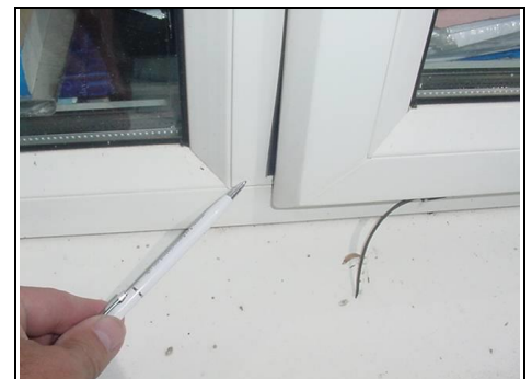
Some double glazed units out of alignment
