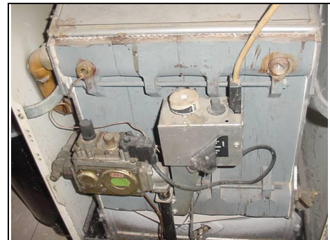
Back of boiler
