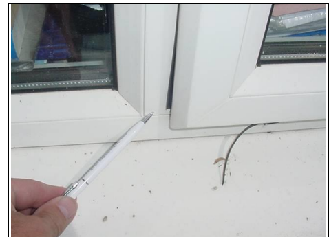
Some double glazed units out of alignment
