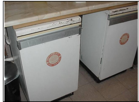
Boilers in kitchen
