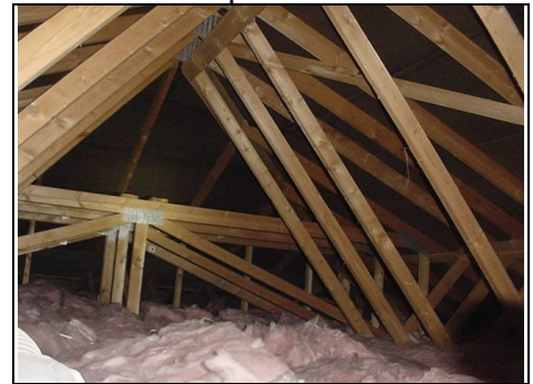
More typical timber thickness in the prefabricated truss roof to the rear left side single storey extension
