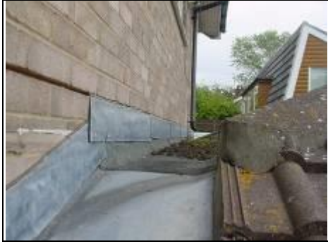
Valley gutter between main building and right side with vegetation
