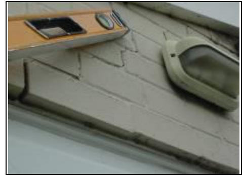
Cracking to front middle
