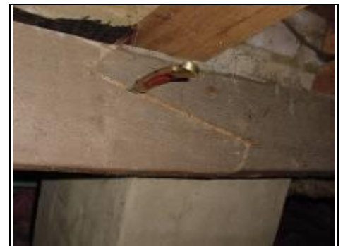
Minor movement to purlins
