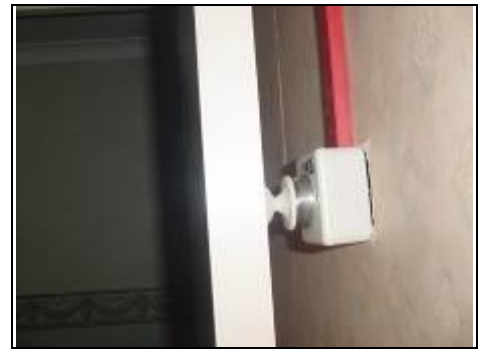
Electric fire door restrainers
