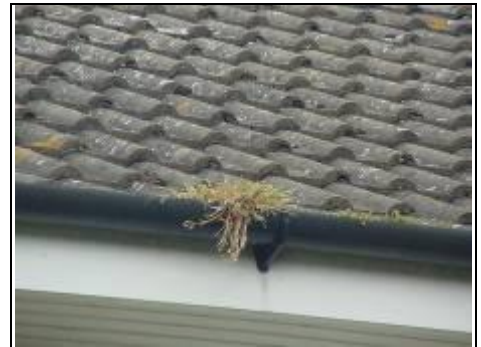
Grass in gutters
