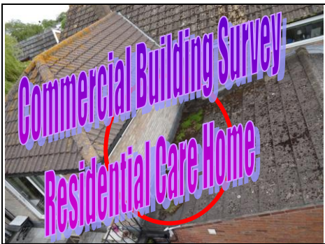
Valley blocked with moss, etc
