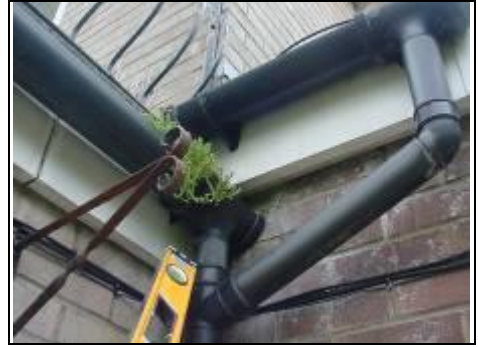
Vegetation growing out of gutters
