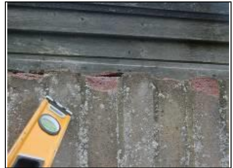
Spalling single brick wall
