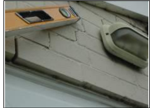
Cracking to front middle
