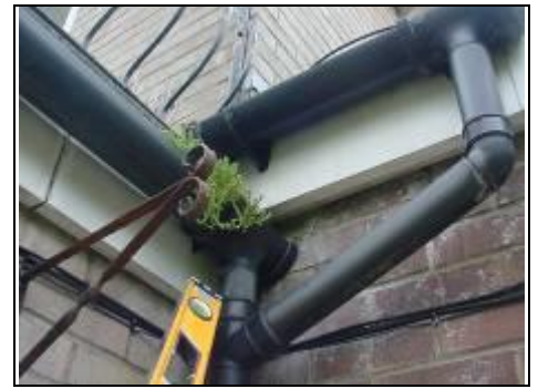
Vegetation growing out of gutters
