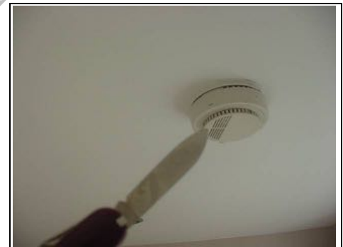
Wired in fire alarm
