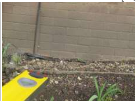
Rainwater hits the ground and bounces back onto the wall
