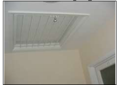
Roof access locked shut
