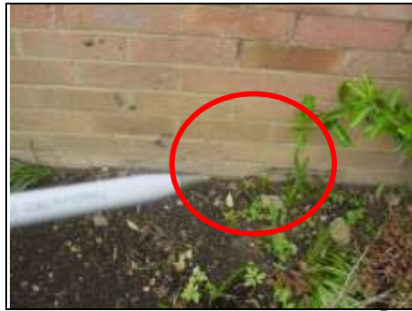
Airbrick almost covered in earth and acting as a gutter
