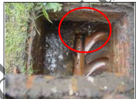
Roots in rear left manhole
