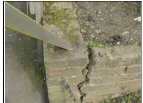
Tree damaged nearby wall
