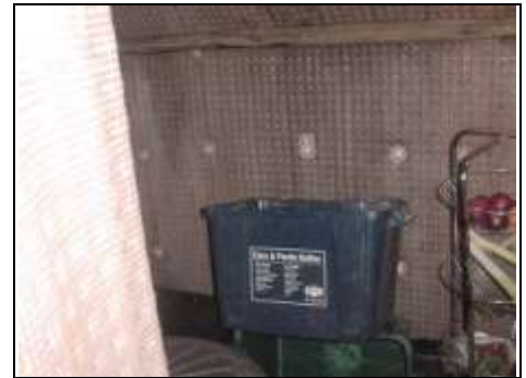
Dampness in under road storage area
