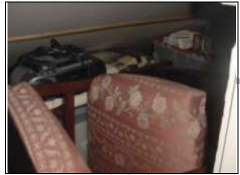
Area to front lined and full of stored items
