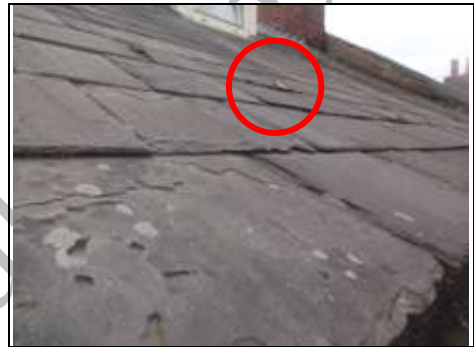
Deteriorating slates (tingle circled)
