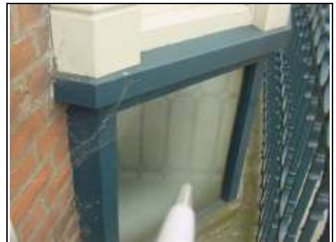
Glazed window to front not to listed building standard
