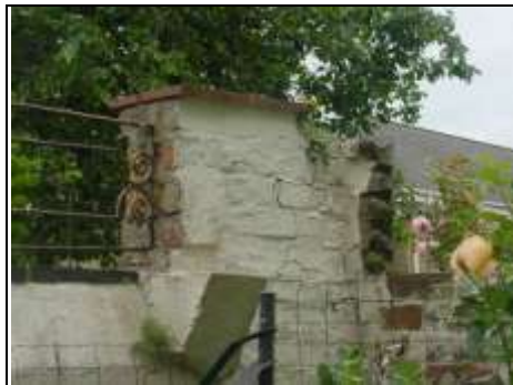
Cracking to wall
