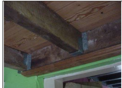
Black mould to timbers
