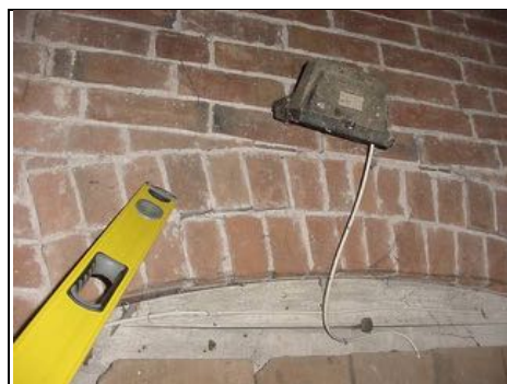
Crack to left gable
