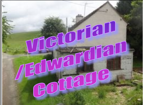
Timber deteriorated to left side
