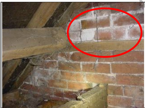
Dampness coming in through walls
