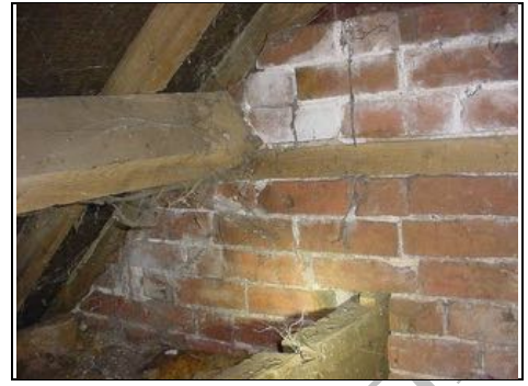
Efflorescence, bonding timber will be affected by dampness
