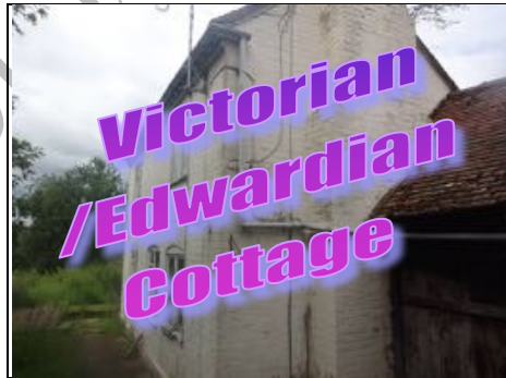
Rear guttering allowing water to discharge down the wall causing moss
