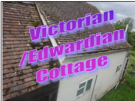
Front guttering needs checking
