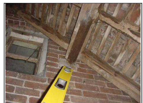
Point load created by purlin has had metal bracket added
