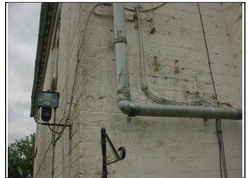
Awkward downpipes to rear left of main house
