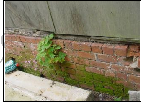
Dampness to rear base of barn due to not having gutters
