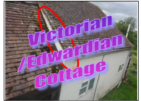
No lead flashing between barn and main building
