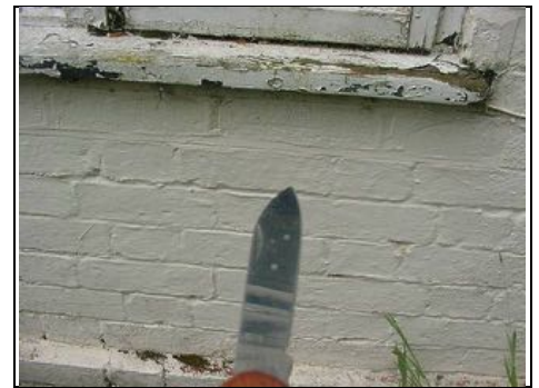
Damage under windows
