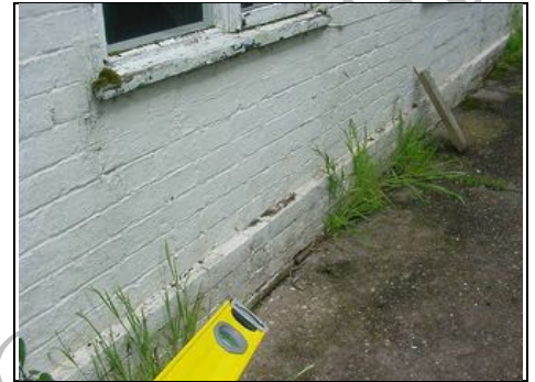
Grass growing against property/dampness
