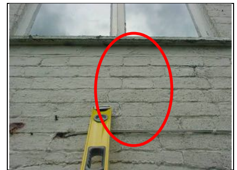
Vertical crack which follows line of mortar
