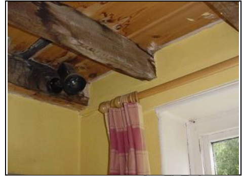
Dampness to timbers in rear lounge
