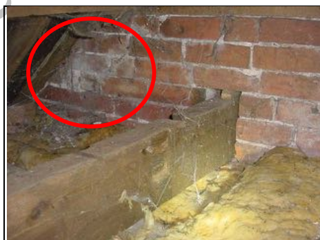
Dampness to right gable
