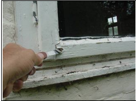
Rot to windows
