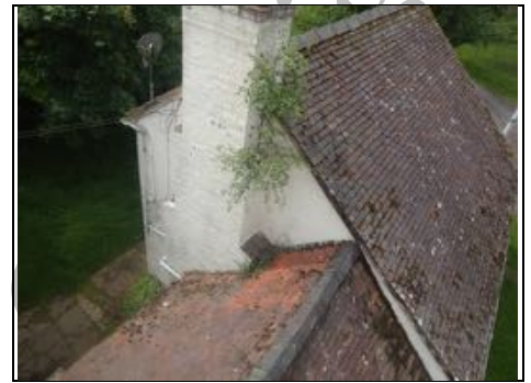
Plants growing out of chimney
