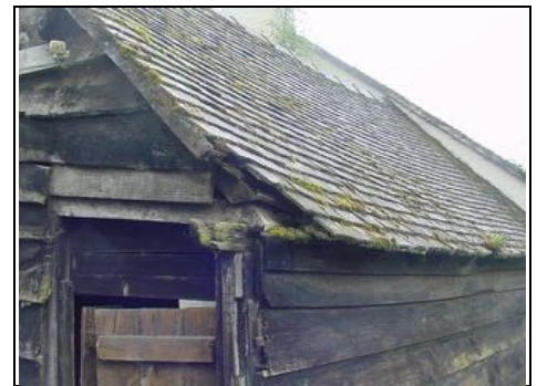
Part missing from barn roof
