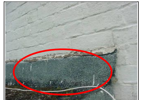
Flashing starting to come away from wall
