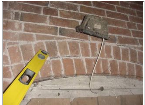
Crack to gable of house visible within the barn
