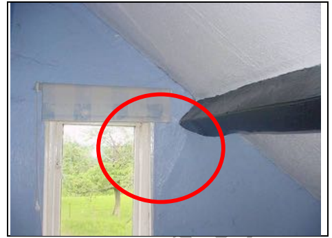
Movement around front window likely to be due to the timber lintel
