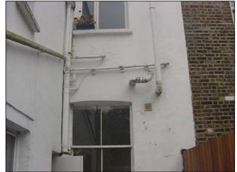
Diagonal cracking to left hand side of window
