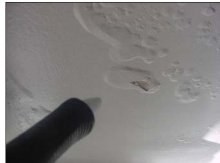
Close up view shows the plastering is starting to fail, as well as the paintwork
