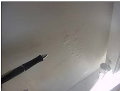
Blistering paintwork in hallway that has been damp proofed
