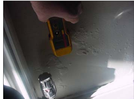
Protimeter damp readings
